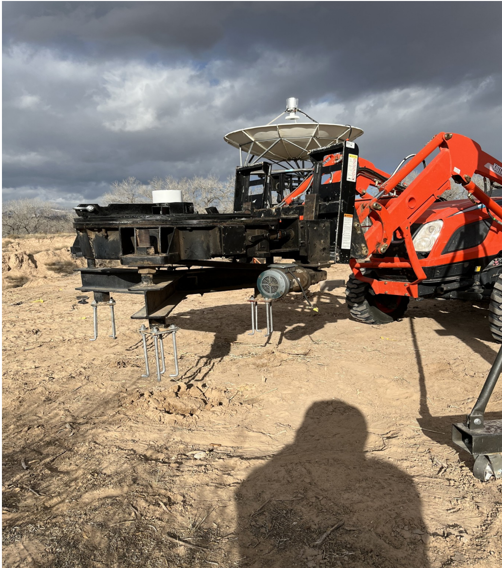
Figure 12. Twelve "J" type anchor bolts are attached to the feet of the AZ mount prior to lowering the mount into its final position over the pier holes.
