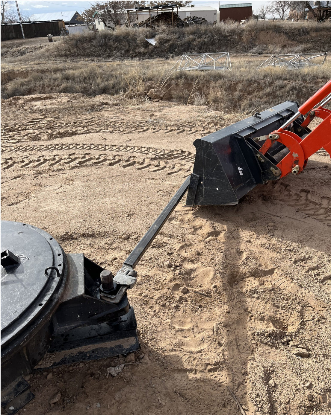
Figure 32. Using a 24" pipe wrench with a steel tube extension and tractor to initially loosen the leveling nuts on the AZ mount.
