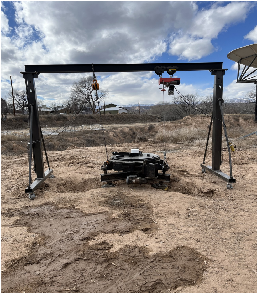
Figure 14. Final concrete has been added to each pier and the mount is leveled and supported by a chain hoist and a cable winch as well as being supported by the center stack of solid concrete blocks until the concrete cures for at least a week (poured 6FEB2023).
