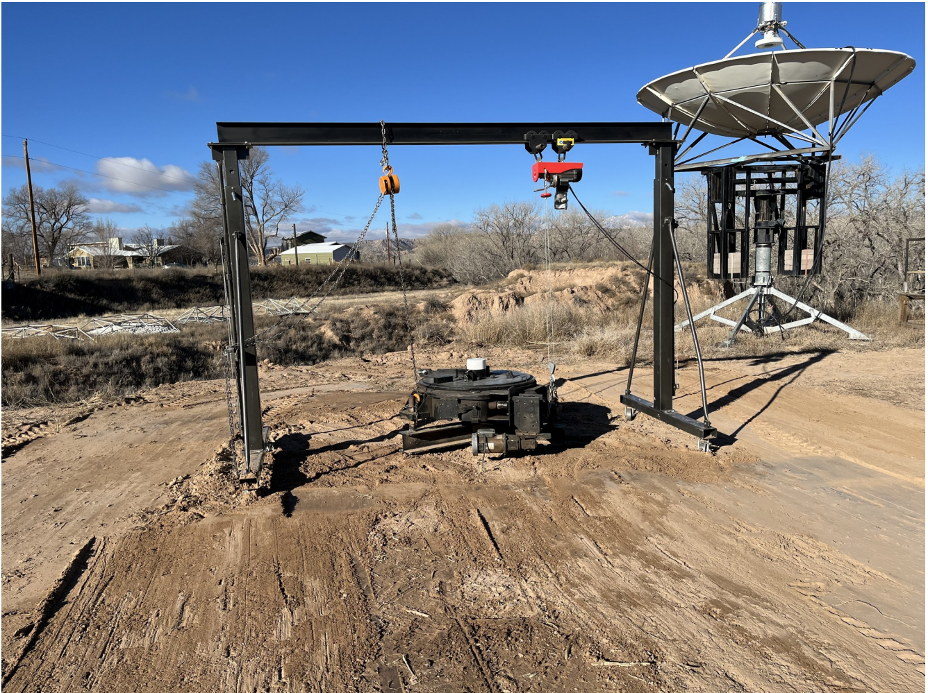
Figure 15. Ground work for the AZ mount installation is now completed (8FEB2023) while curing of the subsurface supporting piers continues. The white cap is a temporary weather-protection measure for the AZ encoder.
