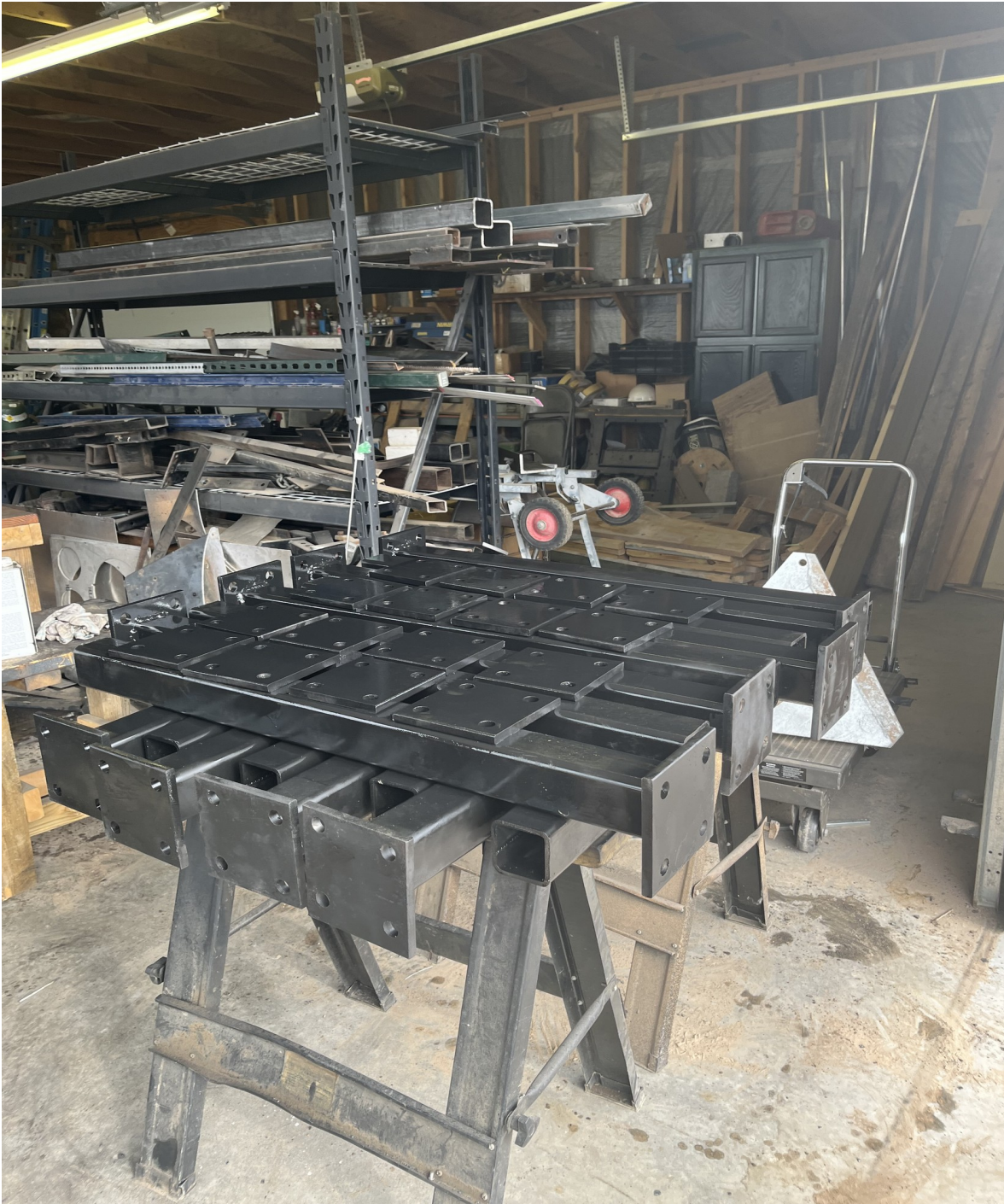
Figure 28. All 16 support posts and 16 top rail plates have been fabricated and painted and are now ready to assemble with galvanized threaded rods (18FEB2023).
