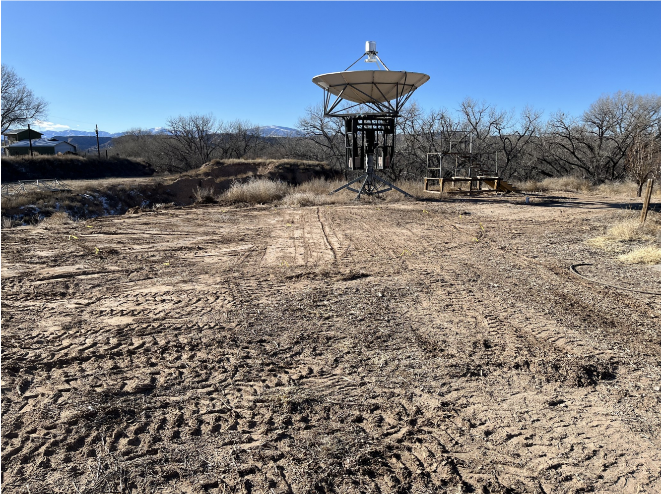
Figure 7. Site where the new ground level AZ/EL mount will be located, shown before construction began on Jan 23, 2023.
