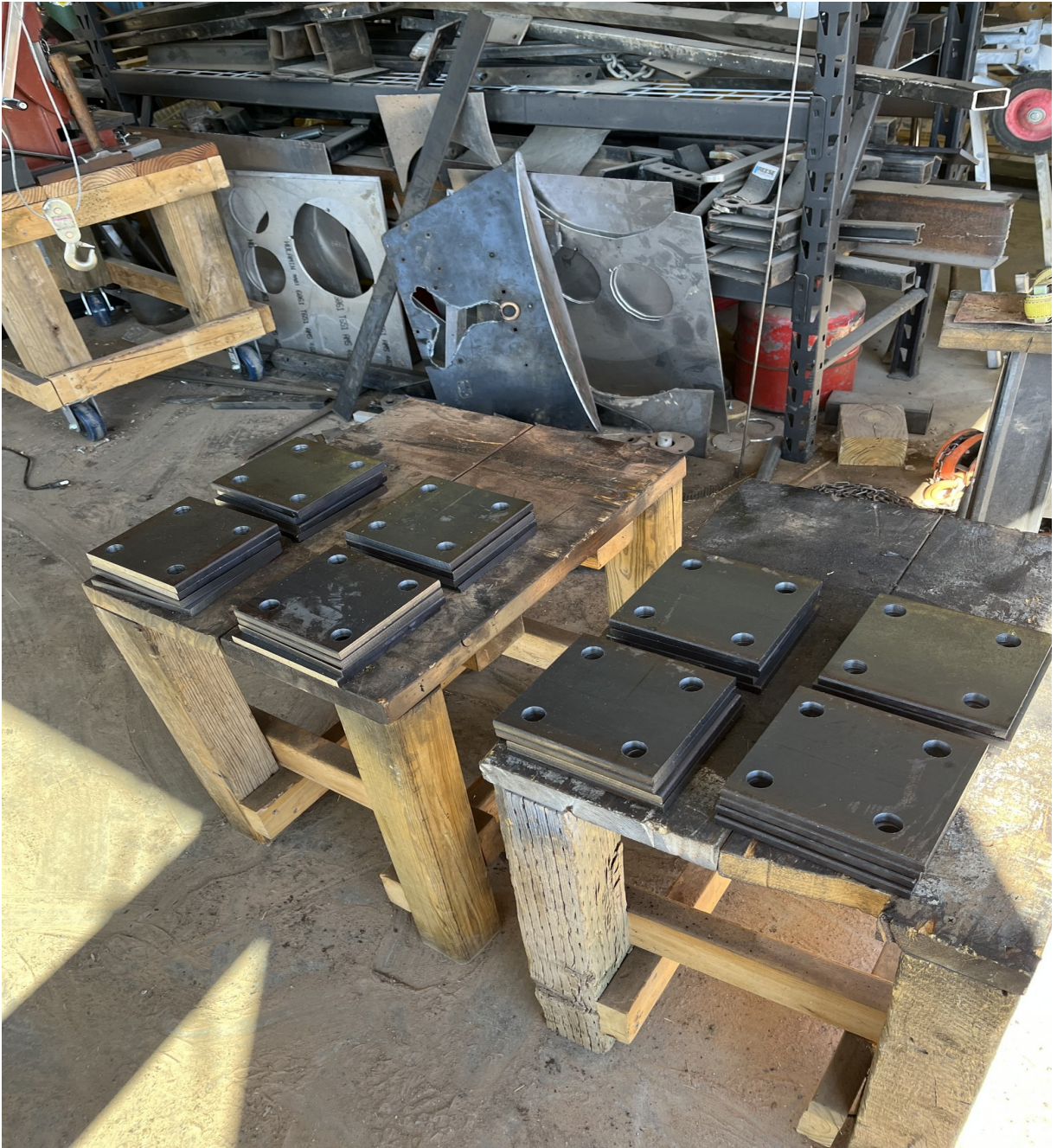
Figure 23. All 32 flange plates have now been bored with four 13/16" diameter holes through each plate and cut to a 6"x6" size.
