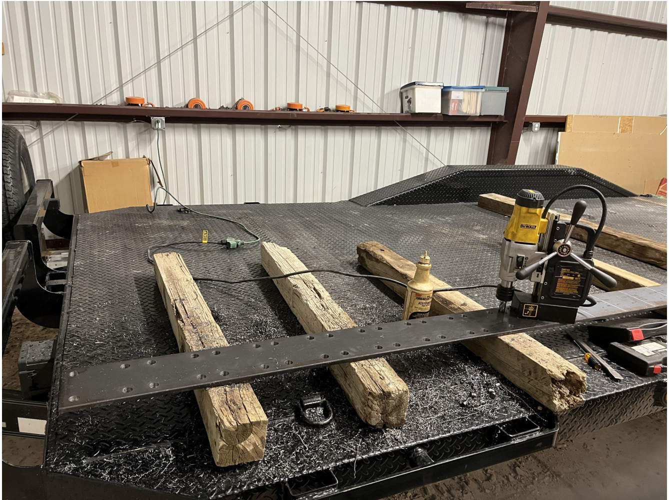
Figure 20. Holes for the threaded rods are bored into a 6" x \frac{1}{2} " x 20' steel bar as part of the fabrication process for the 32 6"x6" support plates for the circular rail (14FEB2023).
