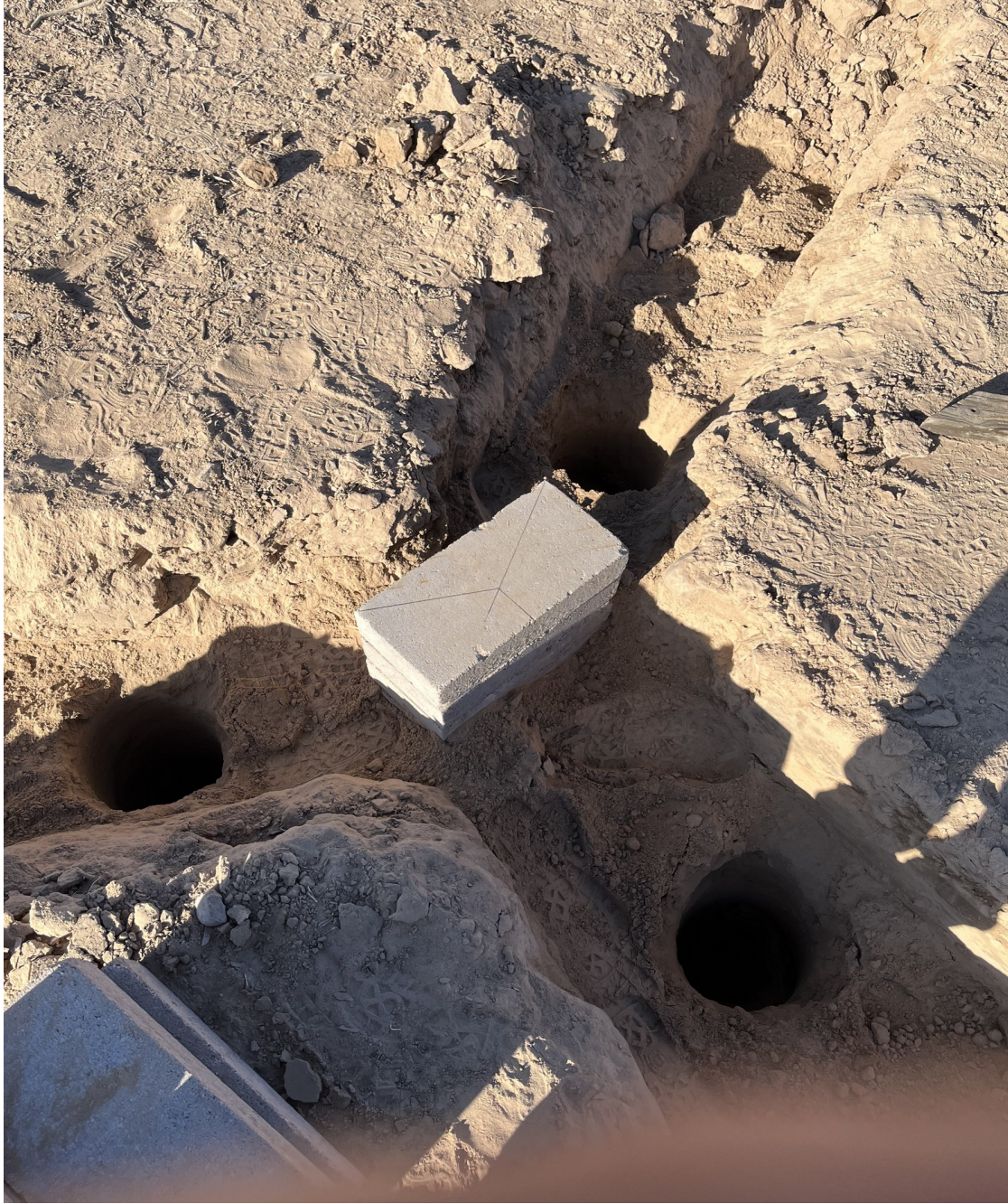
Figure 8. Initial excavations, pier holes, and a center support block stack are shown in preparation for the AZ mount installation.
