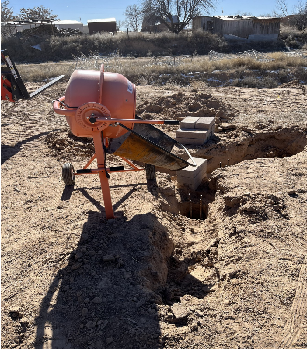
Figure 11. Concrete mixer in position to partially fill each pier hole prior to positioning the AZ mount feet into the holes.
