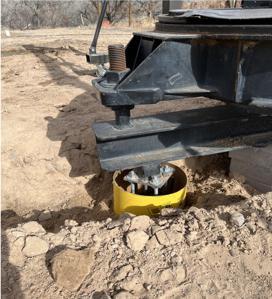
Figure 13. Cardboard forms are placed over each pier hole and the AZ mount is lowered into its final position prior to adding the final amount of concrete to the piers.
