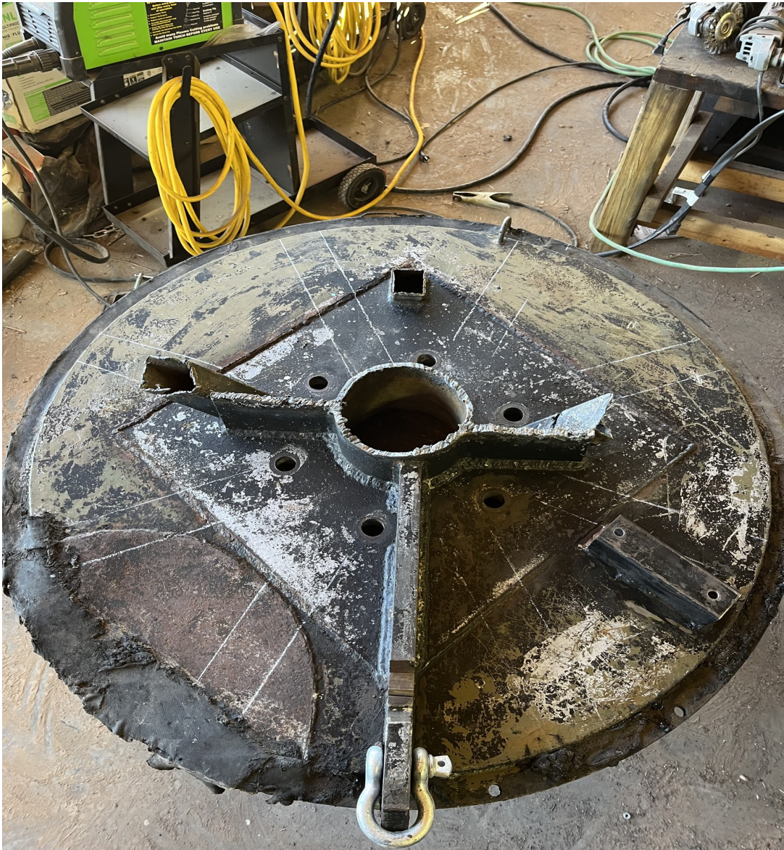
Figure 4. Original top section with unnecessary/interfering structures crudely cut from it.
