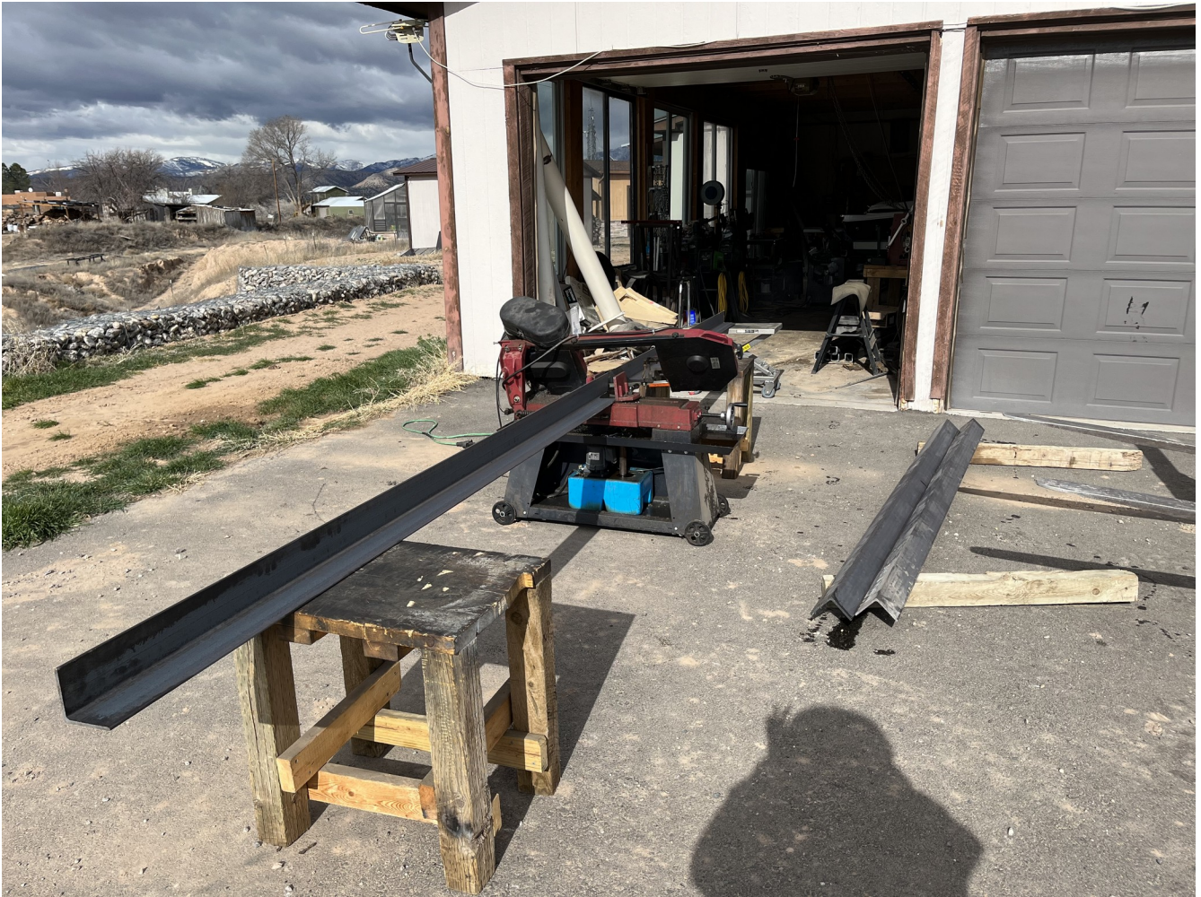
Figure 2. Ten foot long end pieces are being cut from a twenty foot long angle steel piece.
