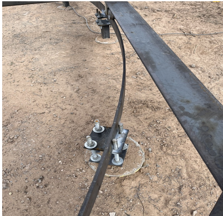
Figure 37. The outside-top nuts and washers on this support post were removed as shown to allow more room for the floating rail to shift as needed to keep wheels on the circular track during rotations.
