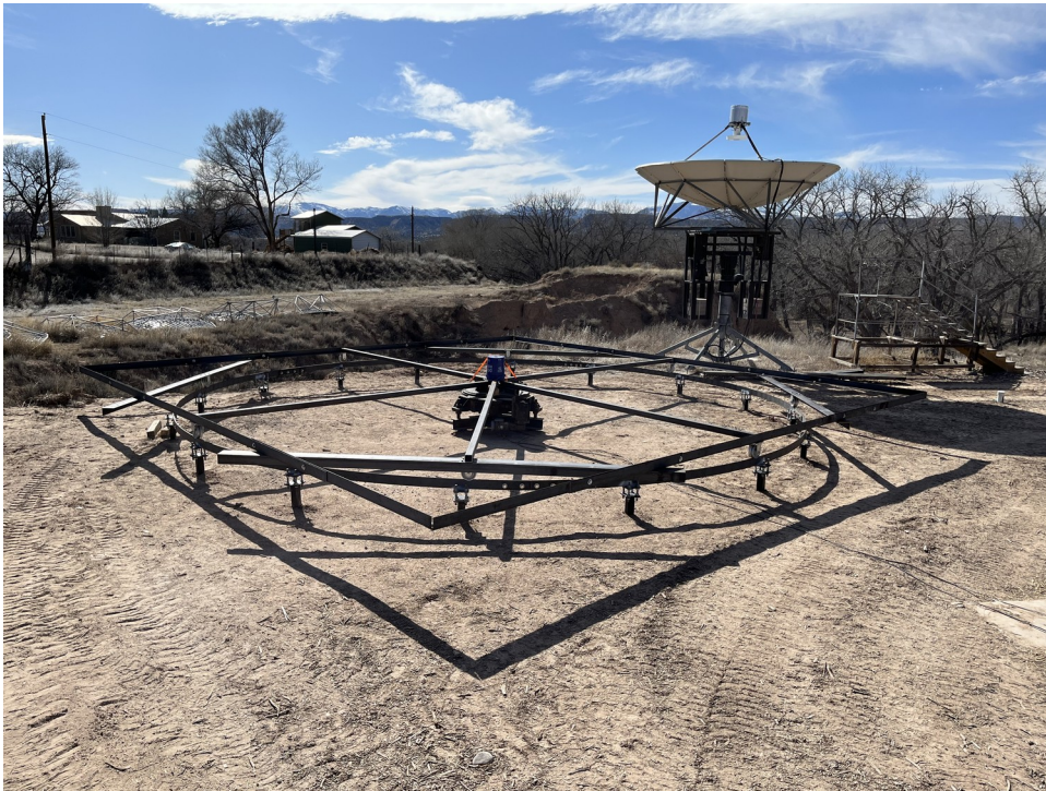
Figure 16. All cross pieces and wheel assemblies are installed onto the circular rail (1APR2023).
