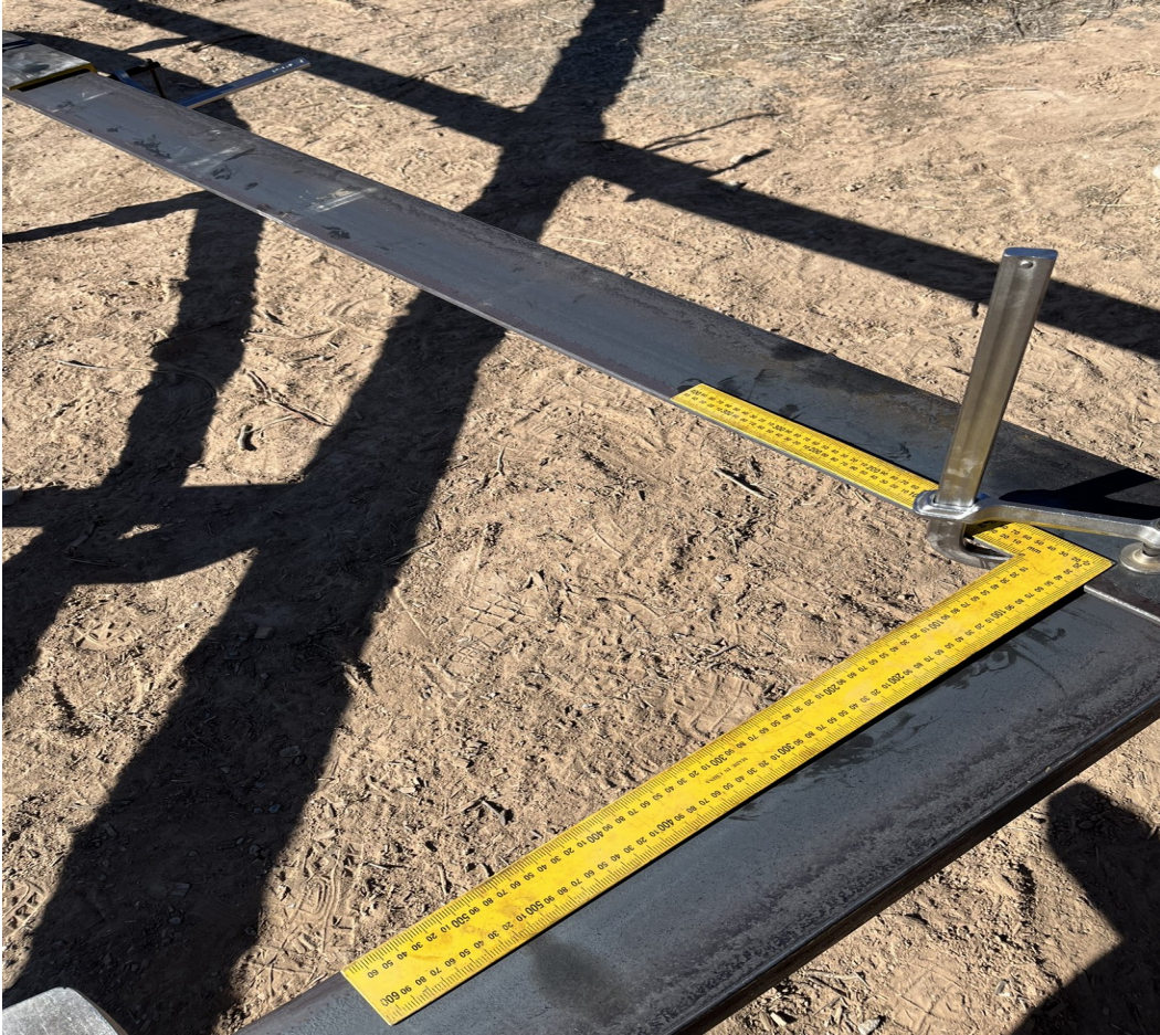
Figure 20. The final corner of the base structures is checked to ensure that it is square before holes are bored and beams are bolted together.
