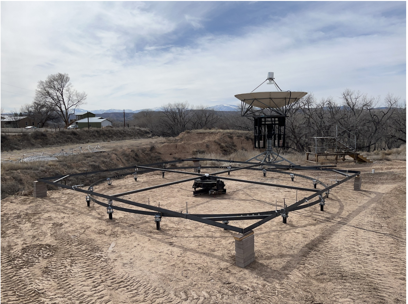
Figure 9. Components of the first half of the rotating base structure are in place ready for final fitting to square everything and lock it in place (25MAR2023).
