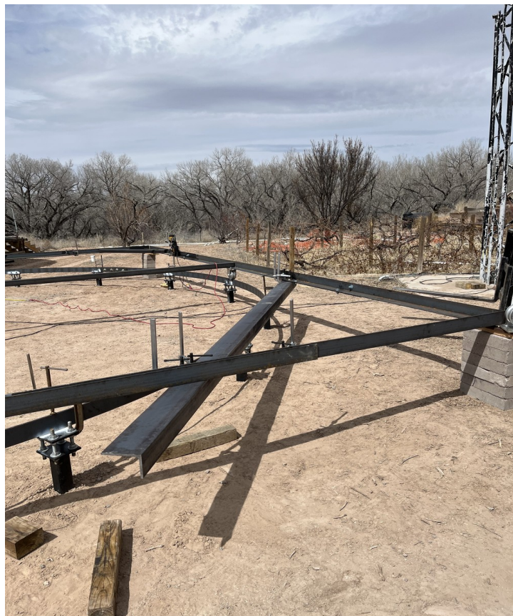
Figure 10. A portion of a 4"x6" truncated square side is clamped into position ready for bolting to the full square structure and mounting of a wheel assembly.
