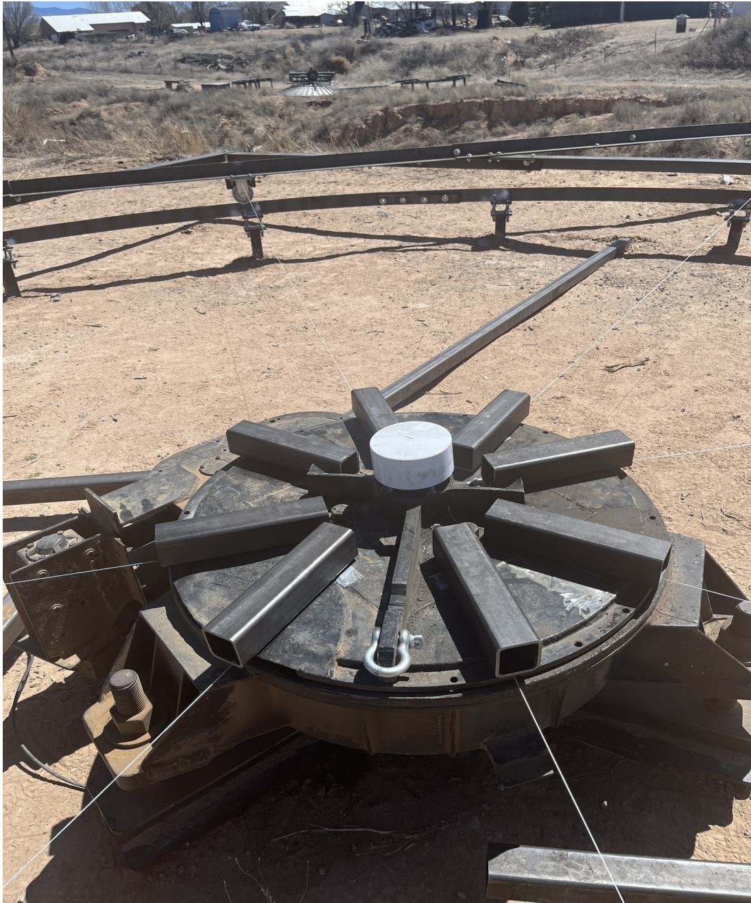
Figure 29. Spoke mounting brackets temporarily positioned on the top plate of the AZ mount prior to cleaning the surface with a rotary brush and welding them in place (6APR2023).
