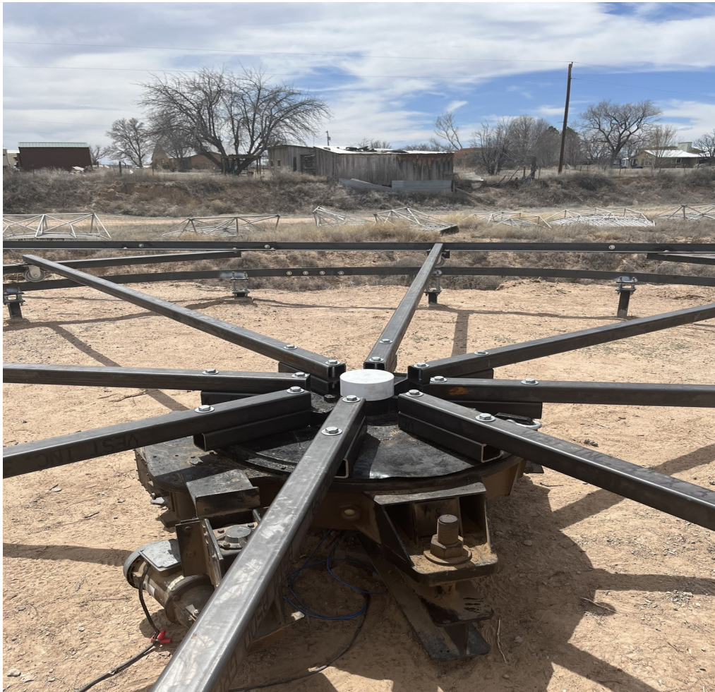
Figure 33. Inward-end spoke brackets are installed onto the spokes and are now ready to be welded to the AZ mount top plate (9APR2023).
