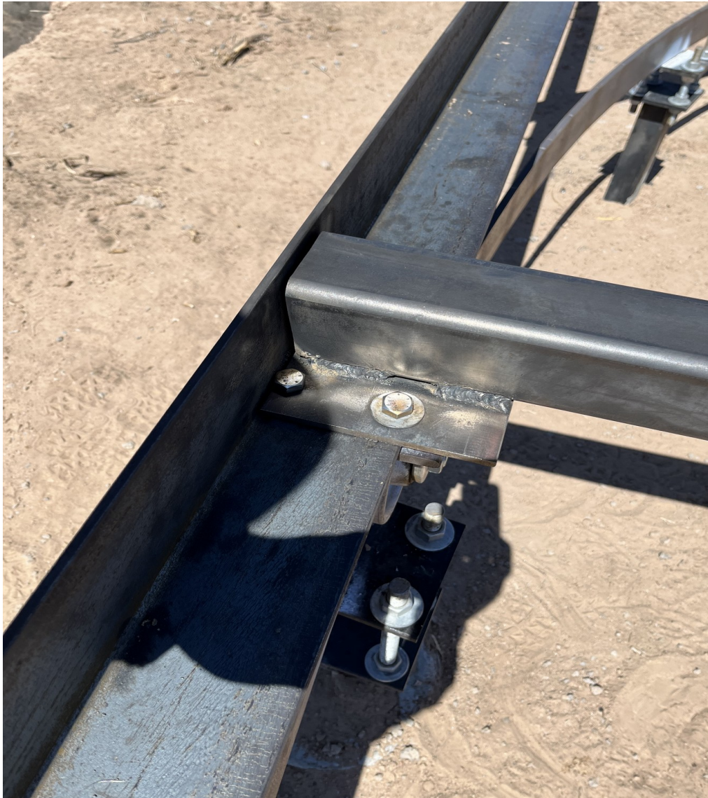
Figure 35. View showing how a spoke flange is welded onto a spoke (10APR2023).
