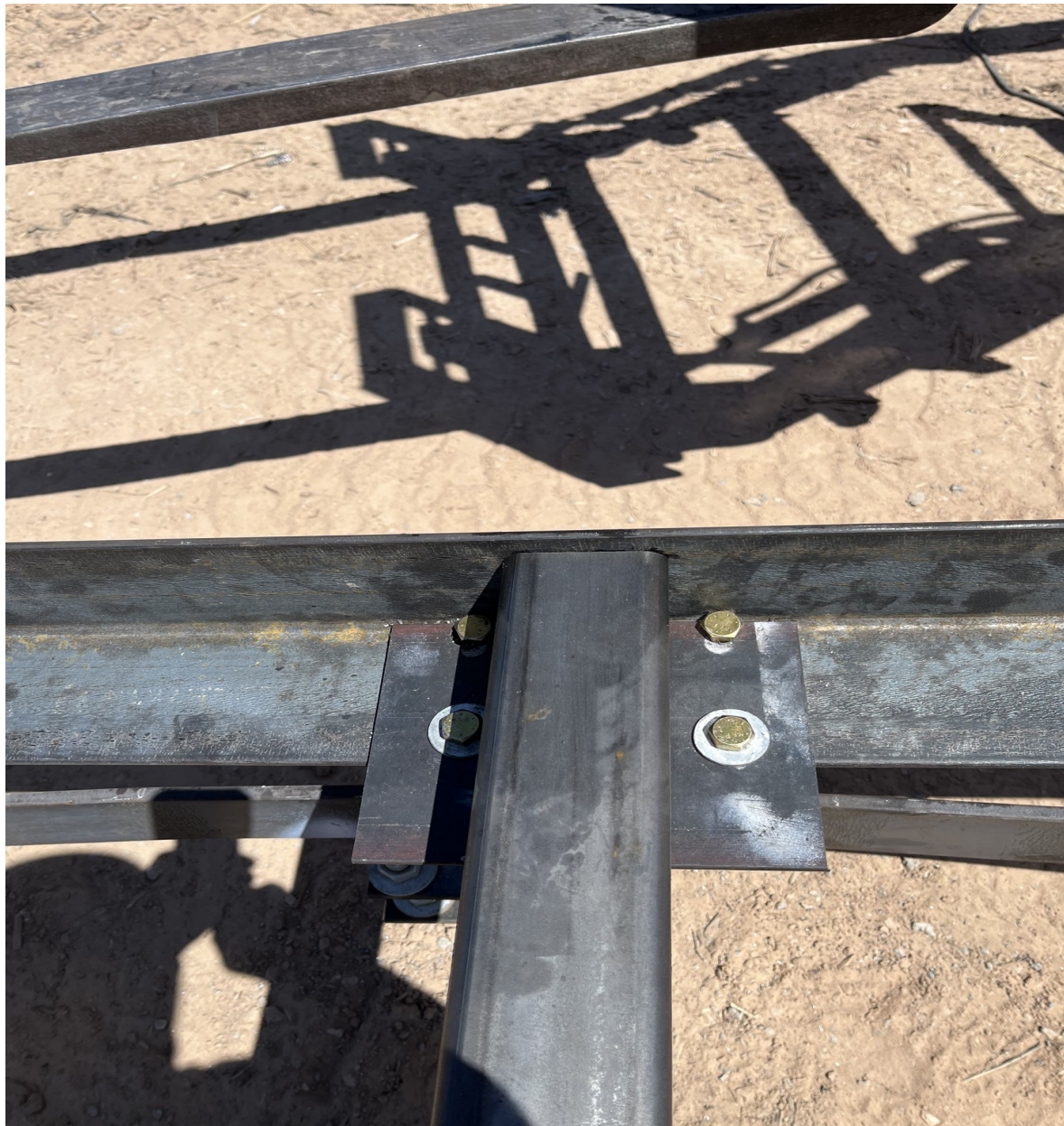
Figure 30. A flange for the full square structure is bolted onto the full square side with its spoke in place ready to be welded to the flange.
