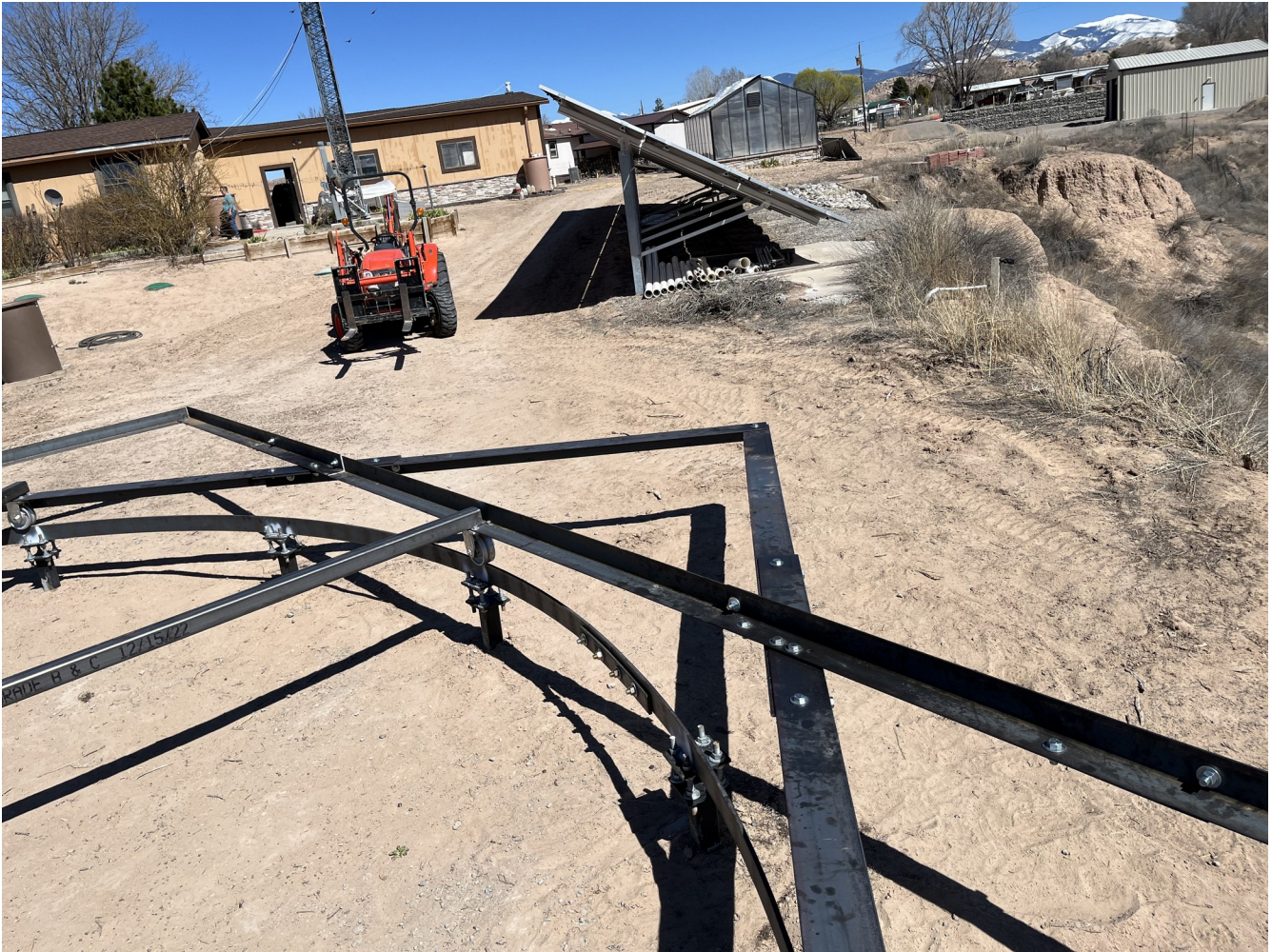
Figure 18. Double hanging bolts are used at the cross over positions for the truncated square corners (2APR2023).
