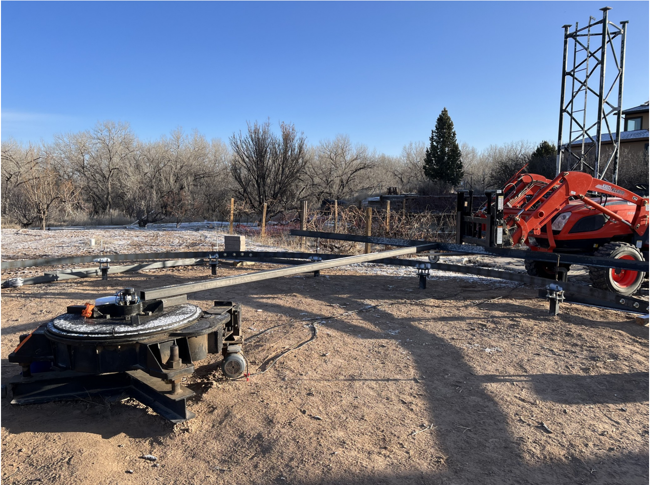
Figure 7. Tractor forks help to put the heavy components into position during assembly of the square rotating base structure.
