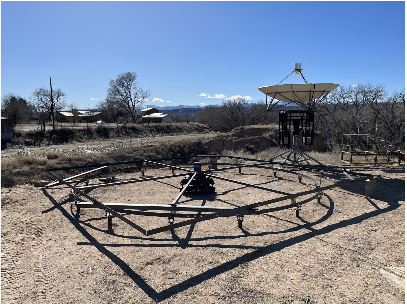
Figure 13. Two of four main cross pieces of the truncated square base structure are now installed (31MAR2023).
