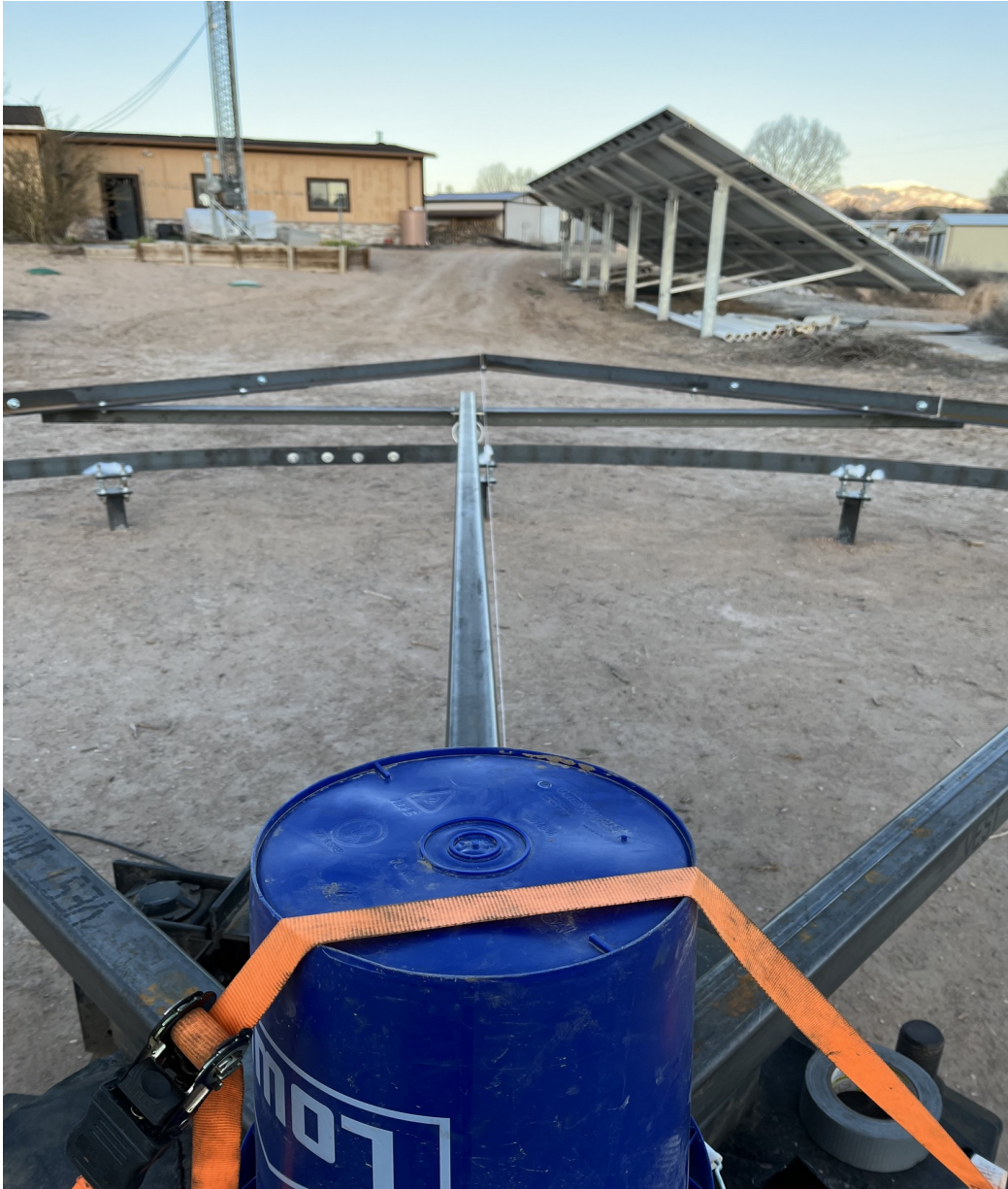
Figure 15. Southeast truncated square wheel position is revealed to be in error by about 2” along the circular rail in the opposite direction from the southwest wheel (31MAR2023).
