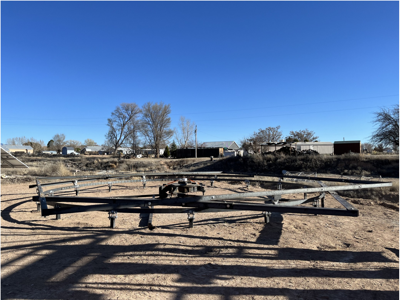
Figure 25. All four wheel spacers are installed on the full square base structure sides (5APR2023).
