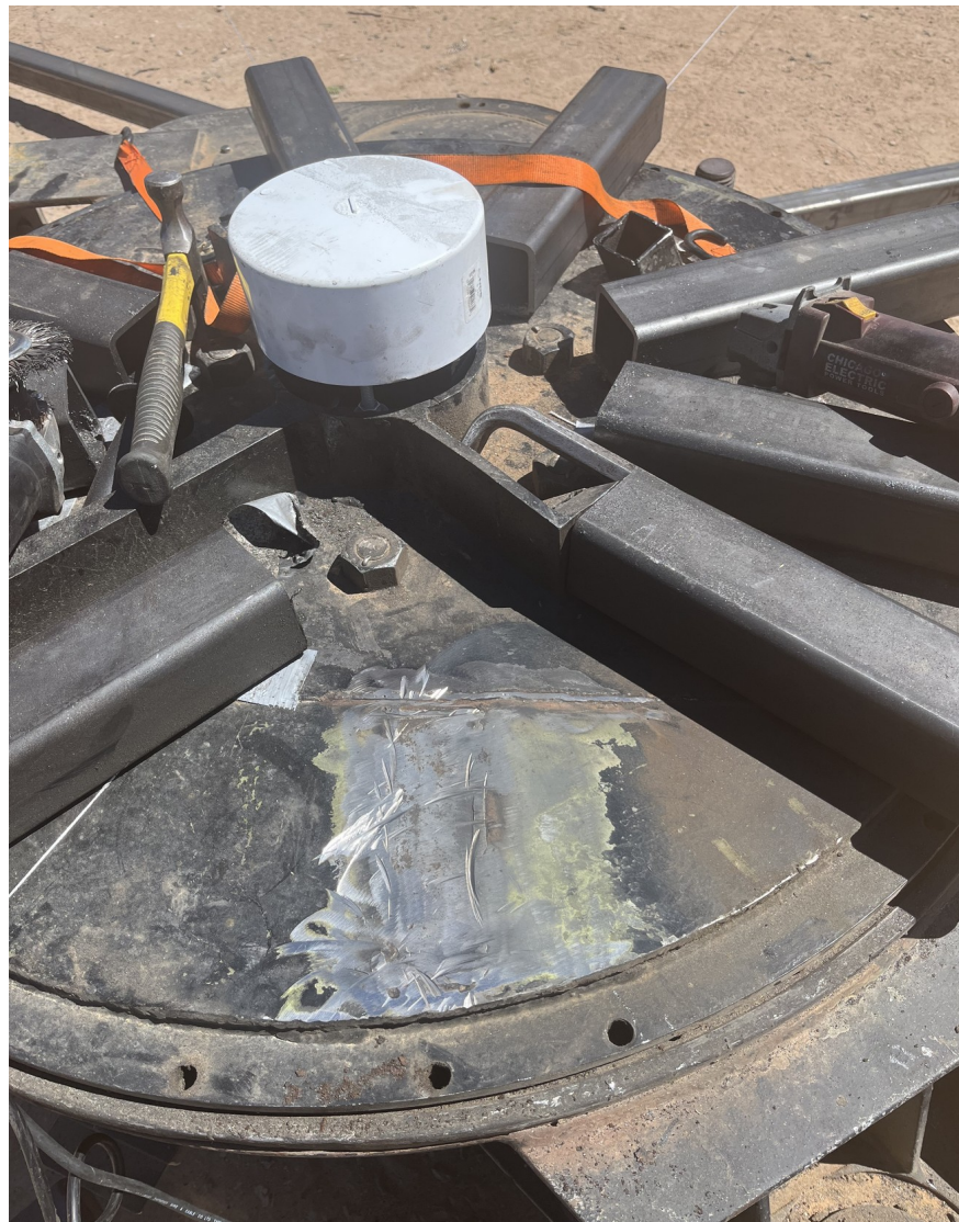
Figure 28. Area where the old bracket was located after removal of the bracket and cleaning with a rotary metal brush.
