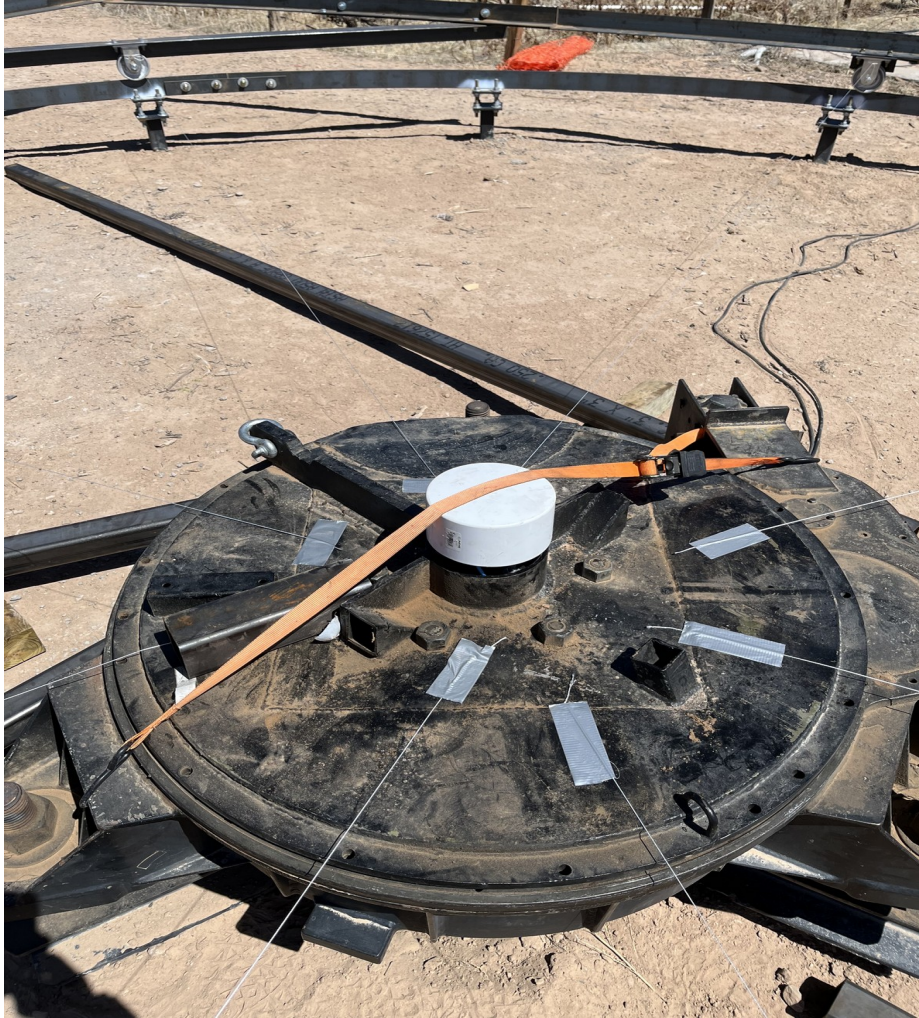
Figure 26. String markers placed on the top plate of the AZ mount to show where spoke mounting brackets will be positioned.
