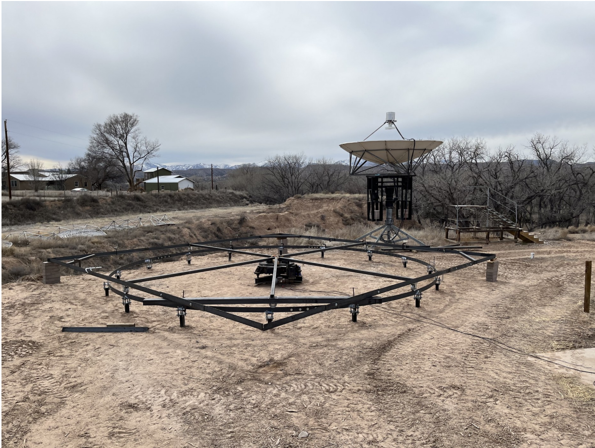
Figure 11. A 15' long portion of a truncated square side piece is shown bolted onto the full square structure and a wheel assembly is shown installed on it with the wheel resting upon the circular rail (28MAR2023).
