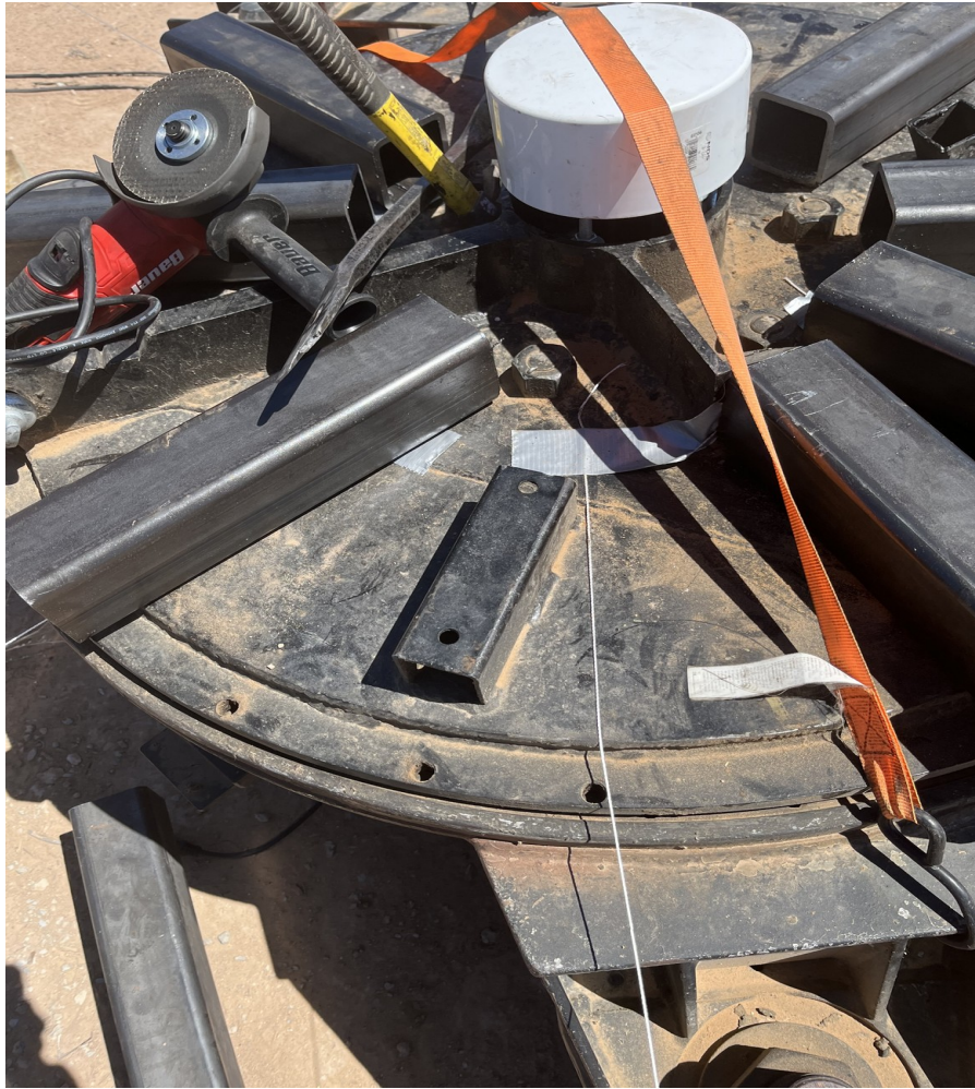
Figure 27. An existing bracket on the top plate (left side of string above) must be removed as its position interferes with the position needed for a spoke mounting bracket whose position is indicated approximately by the string.
