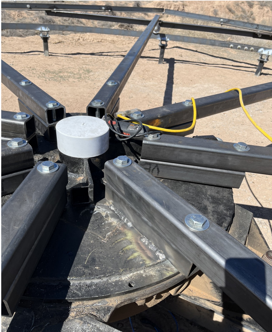
Figure 34. View of how a spoke inward-end bracket is welded onto the AZ mount top plate.
