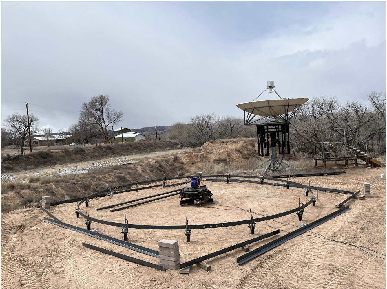
Figure 6. Components of the square rotating base structure are positioned near the circular rail ready to be assembled and installed (24MAR2023).
