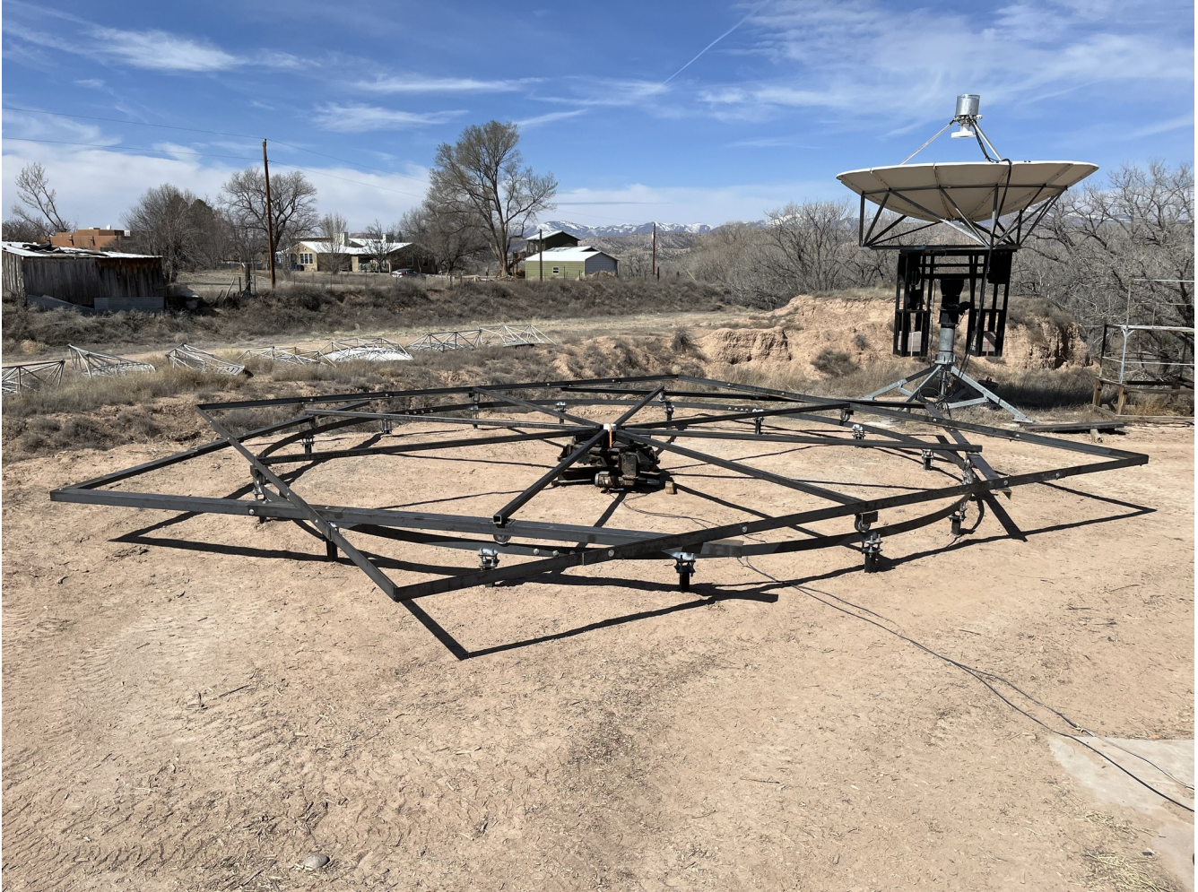
Figure 32. All spoke flanges and brackets are cut and in positions for welding (8APR2023).
