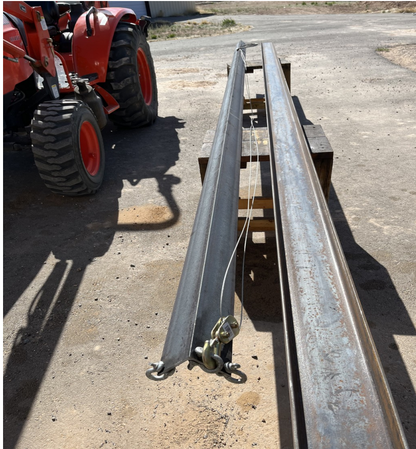
Figure 6. A 20' long angle steel beam is rigged with shackle attachments and a cable pulley to be used as a temporary utility lift beam.
