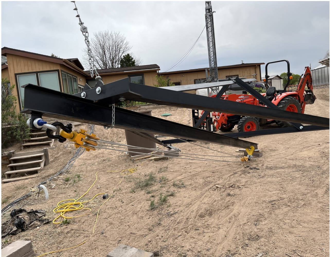
Figure 25. The tripod is lifted partially to allow installation and rigging of the multiple sheaved pulleys.
