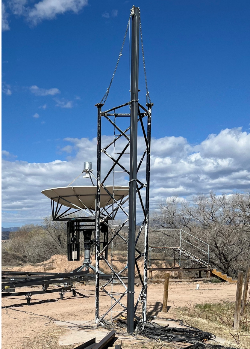
Figure 9. Two support chains are added from the the top of the lift beam to the other two tower legs to increase strength of the lift structure (24APR2023).
