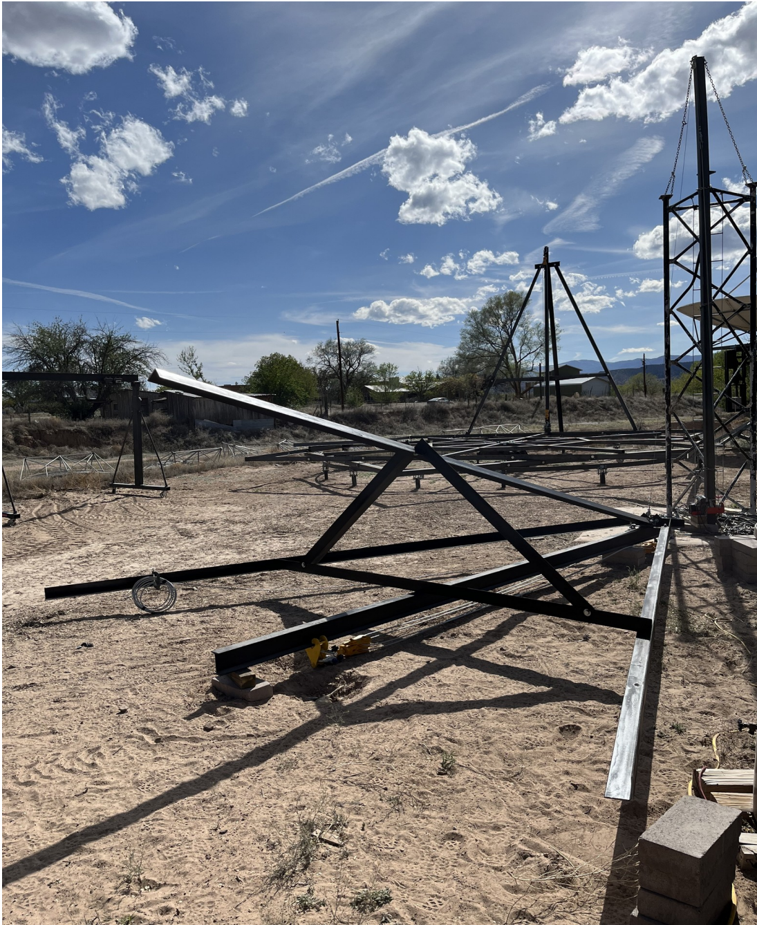
Figure 34. Second lift tripod is fabricated and rigged, ready to be installed on the AZ mount base structure (7MAY2023).
