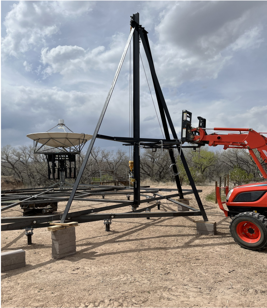
Figure 29. An assembled and rigged lift tripod is positioned onto the AZ rotating base ready for fitting and installation onto the rotating base structure (2MAY2023).
