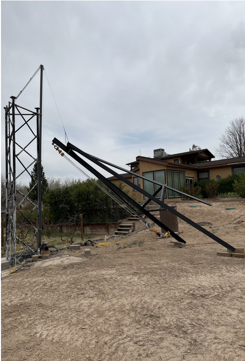
Figure 26. Using an electric cable winch and the utility lift beam to raise the tripod partially.
