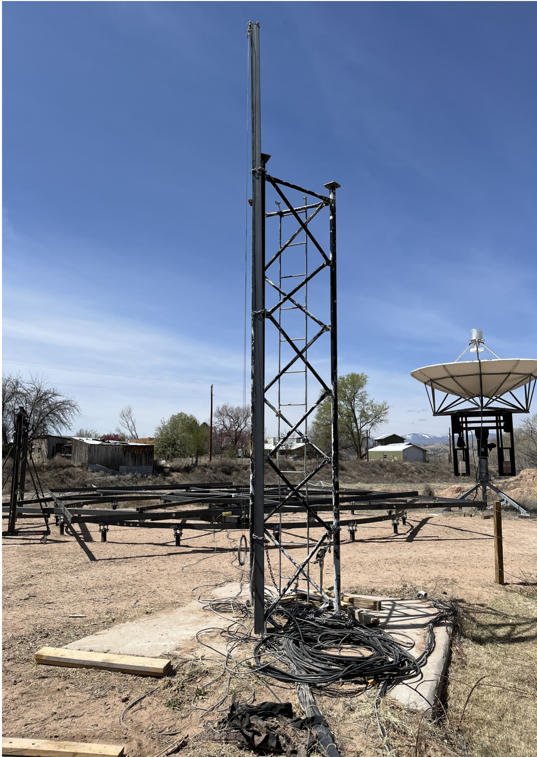
Figure 8. The temporary lift beam is chained into position against one of the tower legs (23APR2023).
