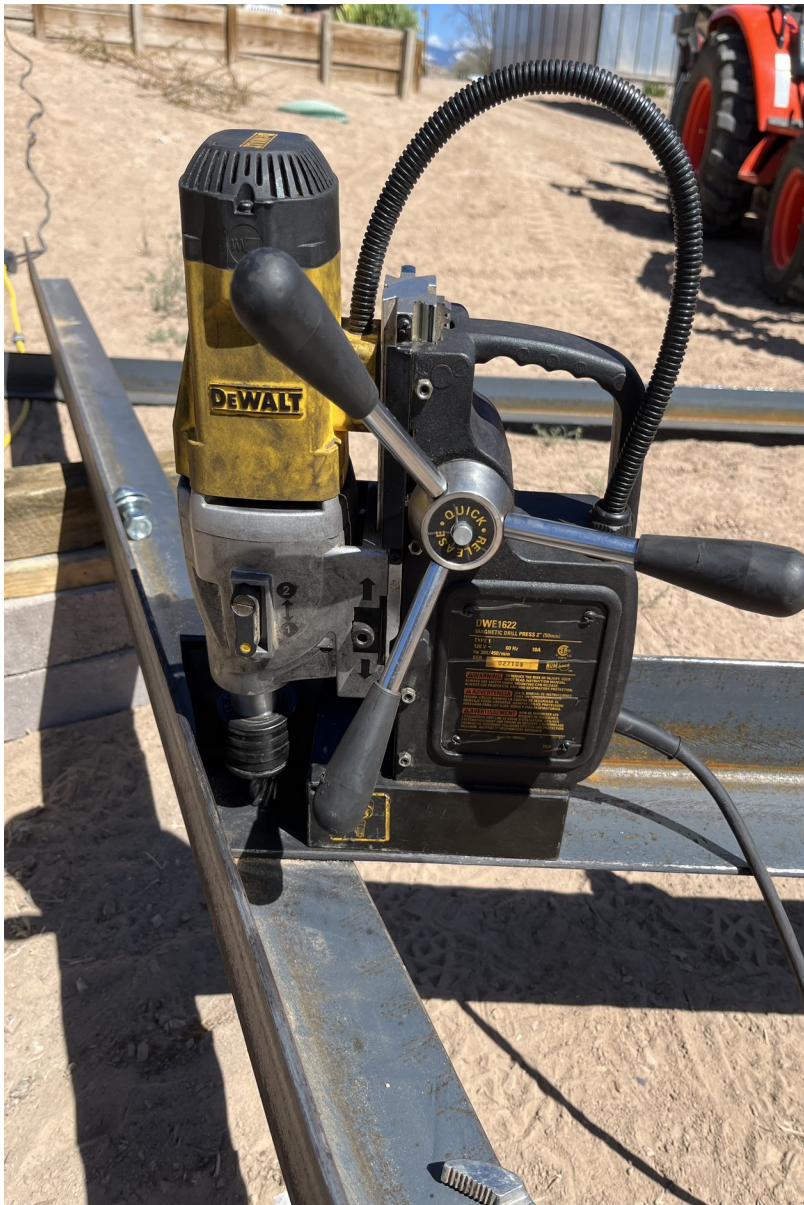
Figure 18. Preparing to bore a hole for a bolt to connect a horizontal tripod member to a sloping side member.
