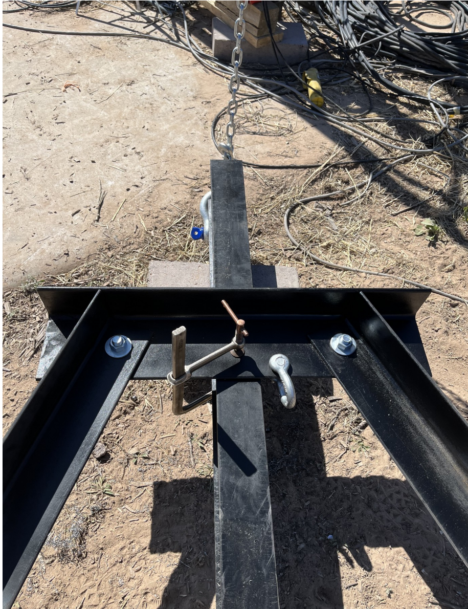
Figure 20. Upper end of the principal side of a lift tripod bolted together (29APR2023).
