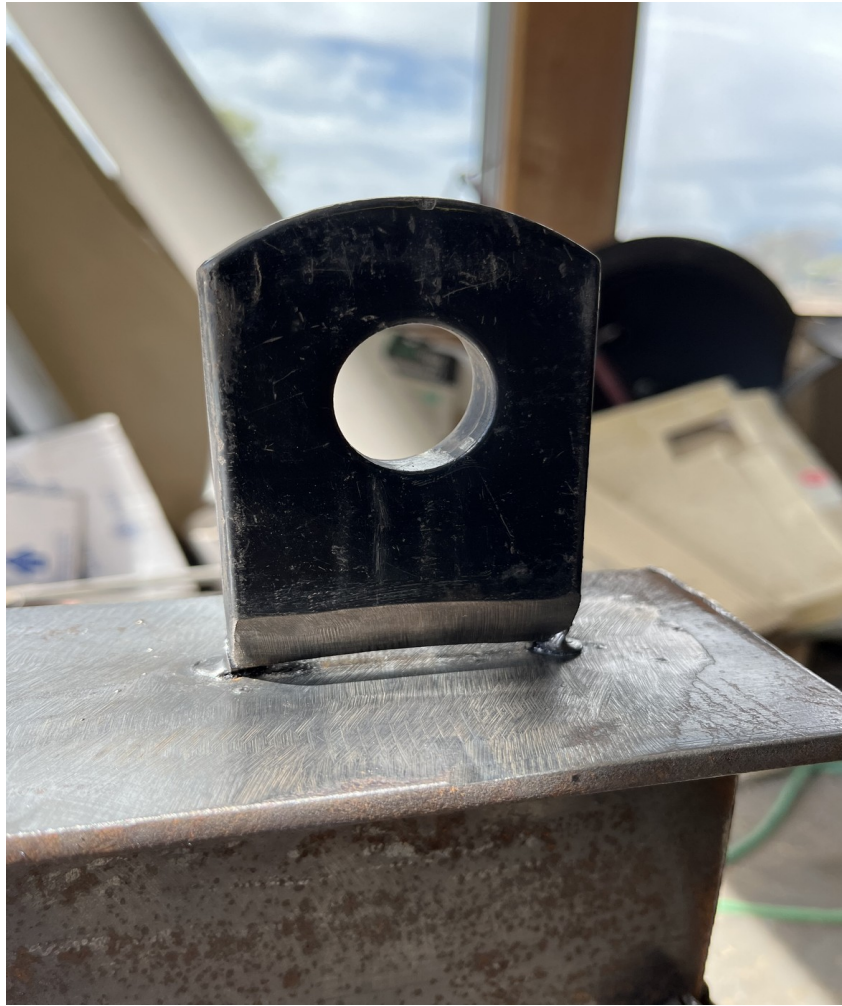
Figure 13. Lifting tab is spot welded in position with a 3/32" gap between the tab and the I-beam.
