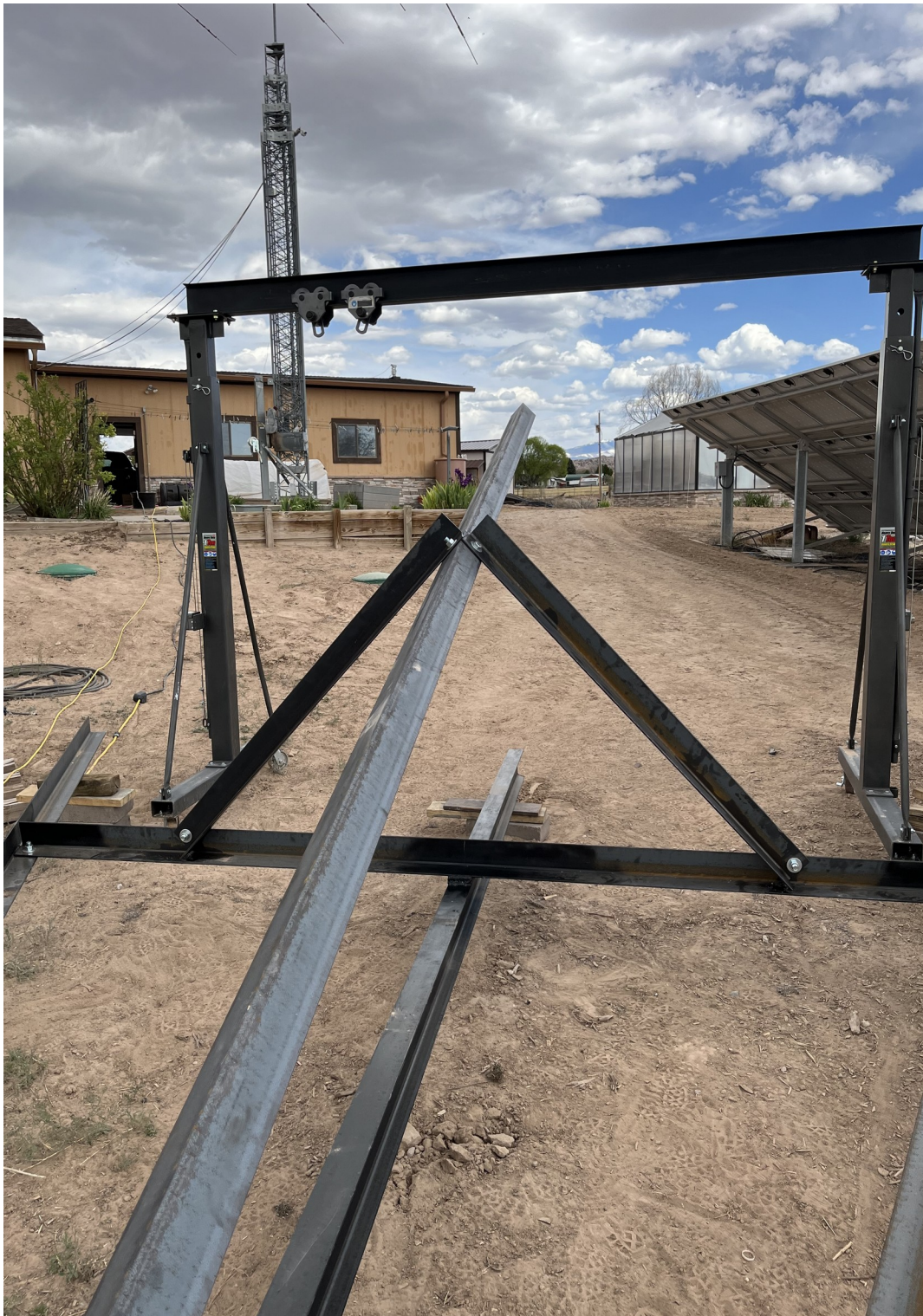
Figure 22. All three cross members are now installed on the tripod structure (1MAY2023).
