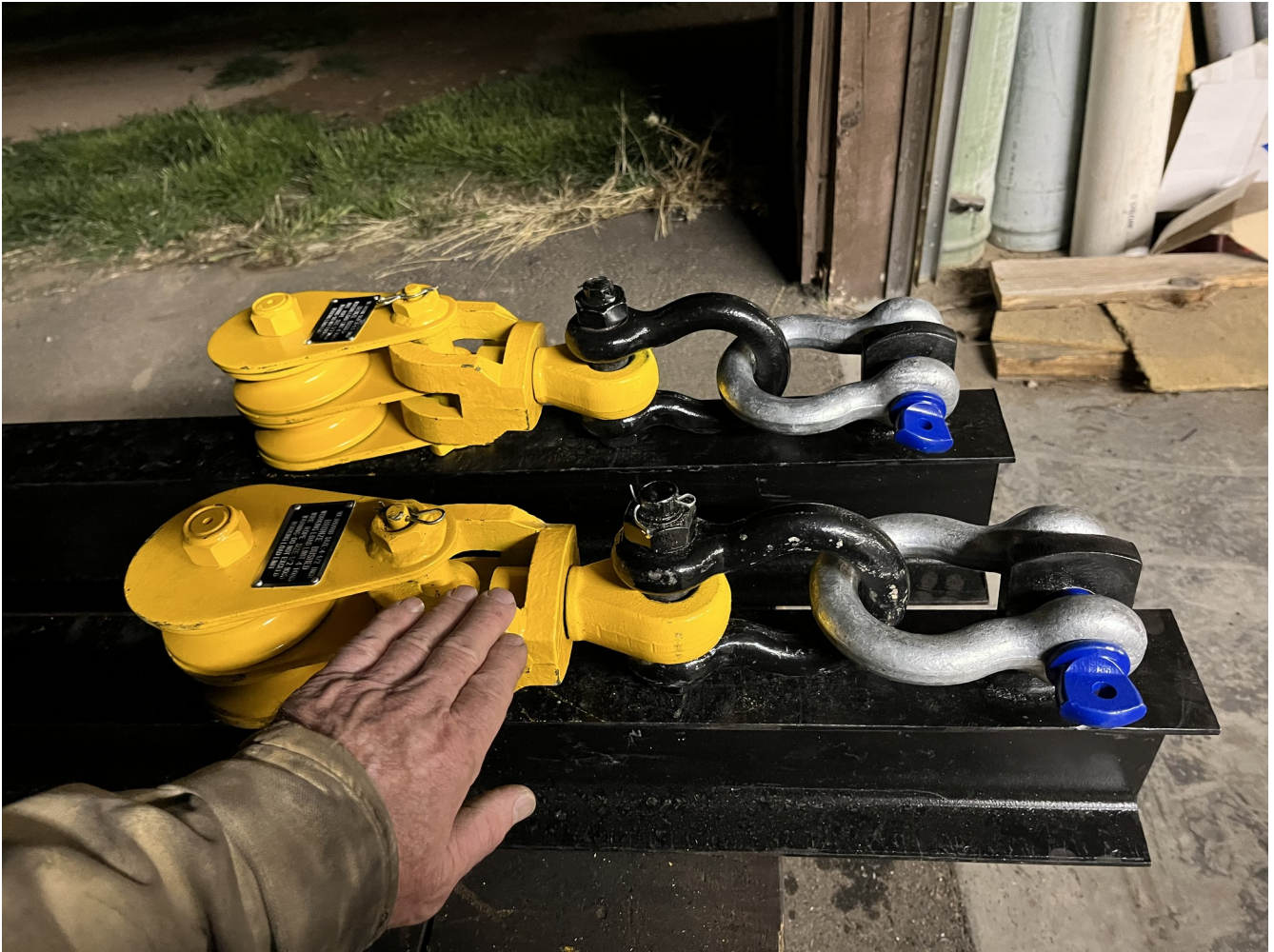
Figure 15. Attachment of the lifting tabs is completed. Upper lifting pulleys are shown in place.
