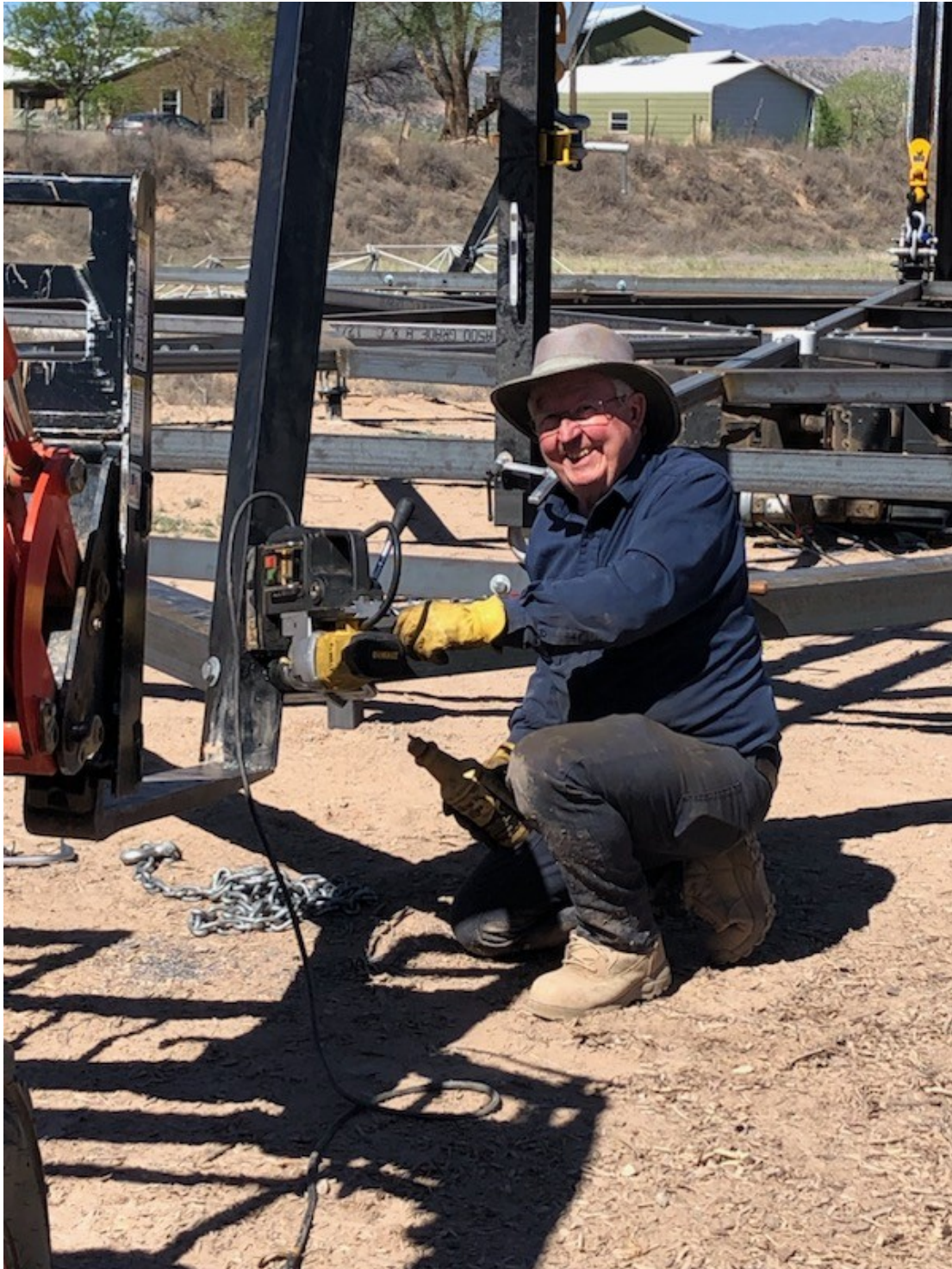
Figure 35. Boring a bolt hole through the auxiliary leg and base frame while installing the second lift tripod (8MAY2023).
