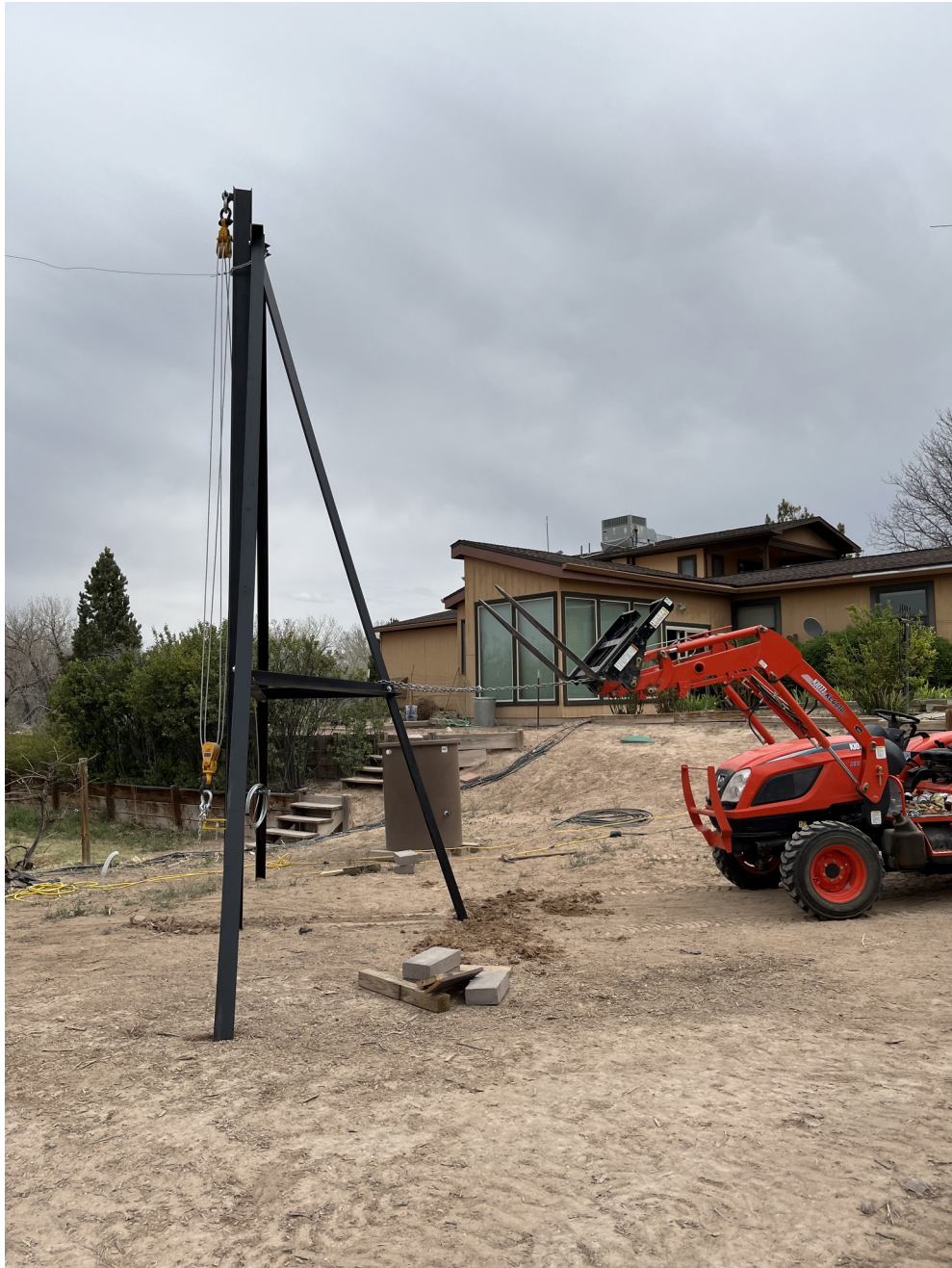
Figure 27. Using a chain and tractor to pull the tripod into a standing position (2MAY2023)
