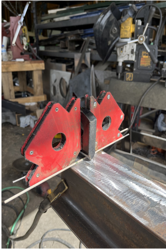
Figure 12. A lifting tab is temporarily spaced above the I-beam surface using two 3/32" diameter welding rods and held between two welding magnets.
