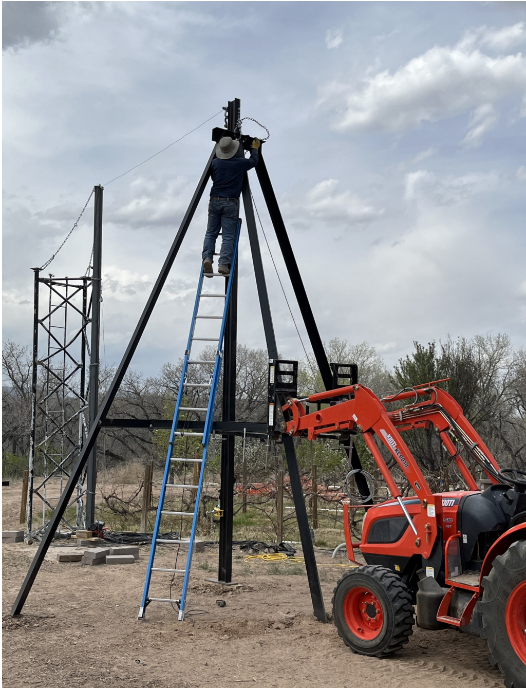
Figure 28. Using an extension ladder to remove the utility lift beam chain and hardware.
