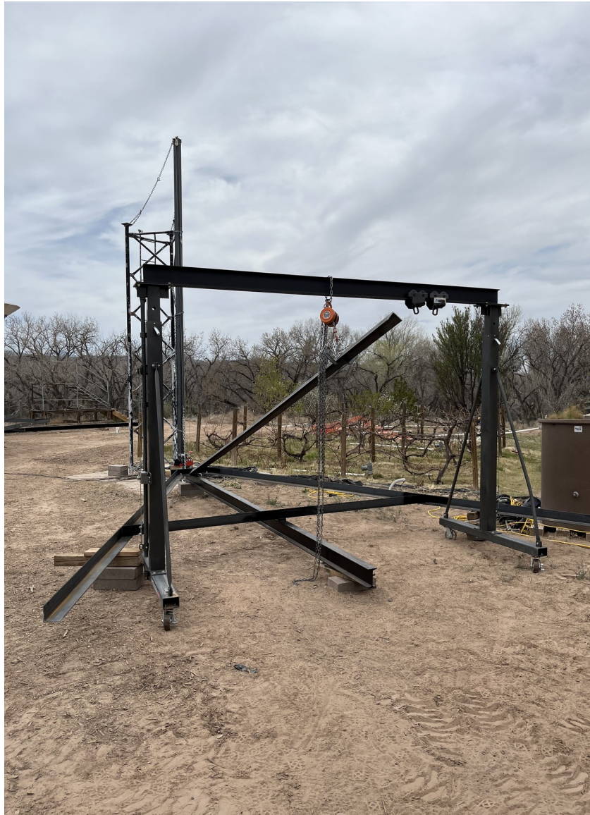
Figure 21. Third leg of the tripod is lifted into position using a chain hoist and gantry (30APR2023).
