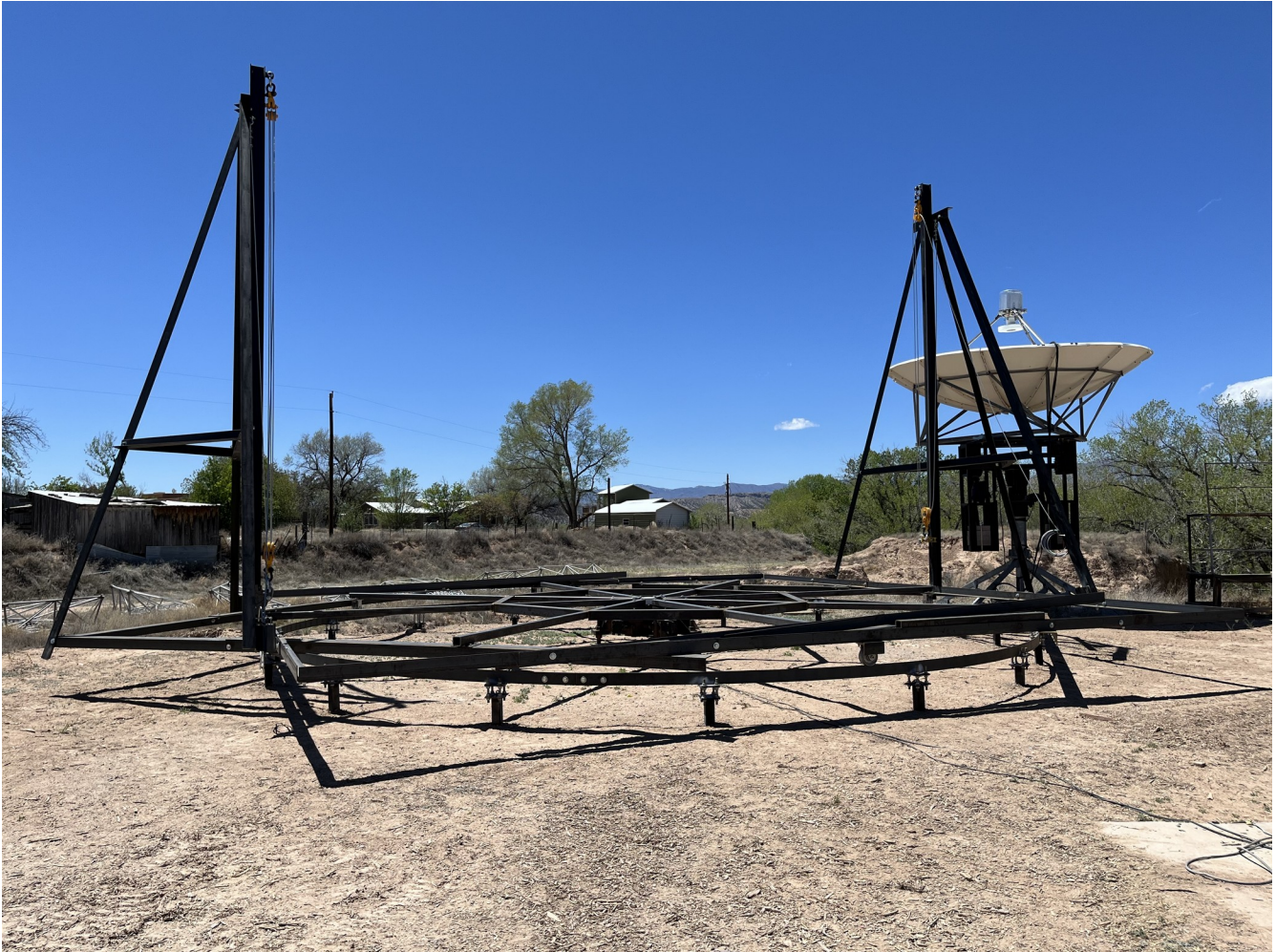
Figure 36. Second lift tripod is installed on the AZ mount rotation base structure (8MAY2023).
