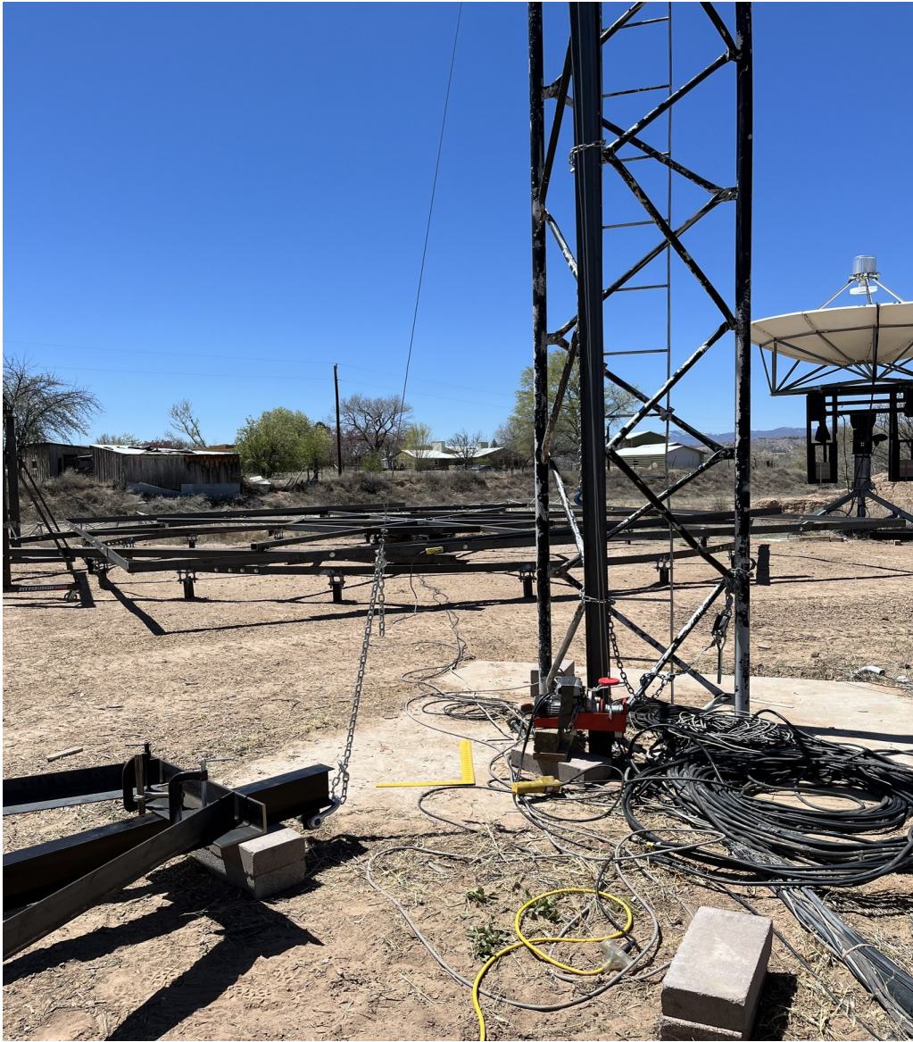
Figure 16. An electric cable winch is shown chained to the base of the tower for use during leveling, squaring, and assembling the various tripod components.
