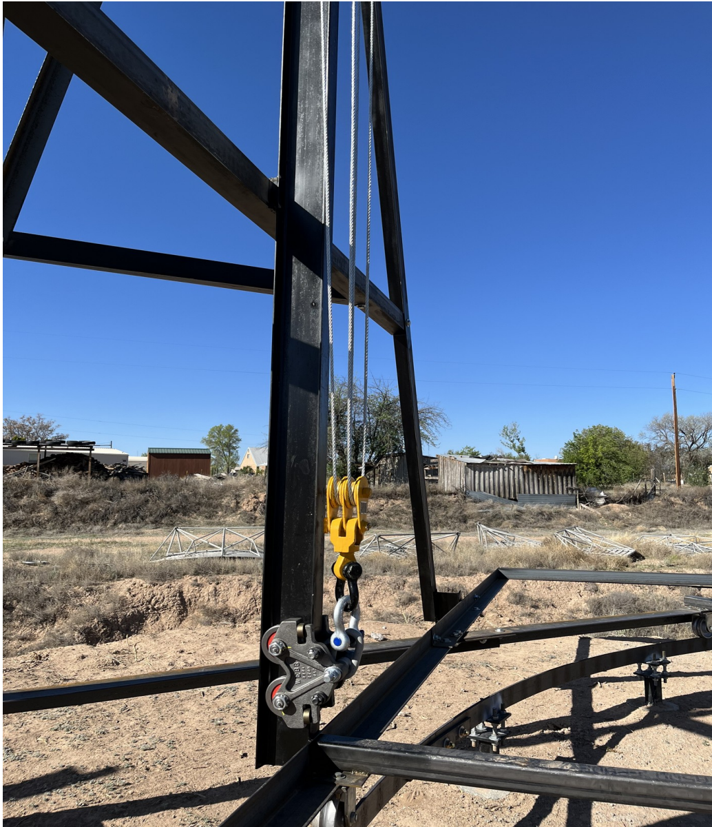
Figure 32. I-beam trolley end of the tripod lift system (5MAY2023).
