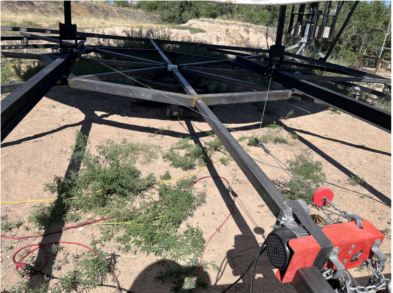
Figure 2. Winch connections for maintenance mode to access negative elevation angles safely (23JUL2023).
