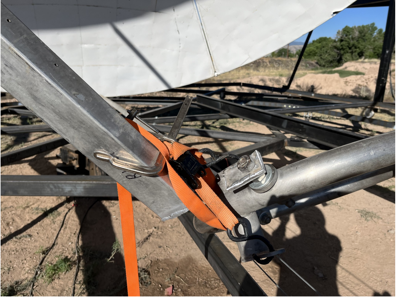
Figure 15. Broken beam end is strapped near the mating piece which is mounted onto the ring (28JUL2023).
