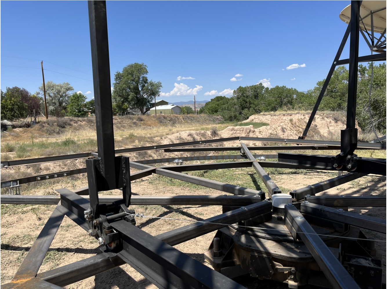
Figure 4. View showing how the maintenance mode cable connection is made to the horizontal trolleys (25JUL2023).
