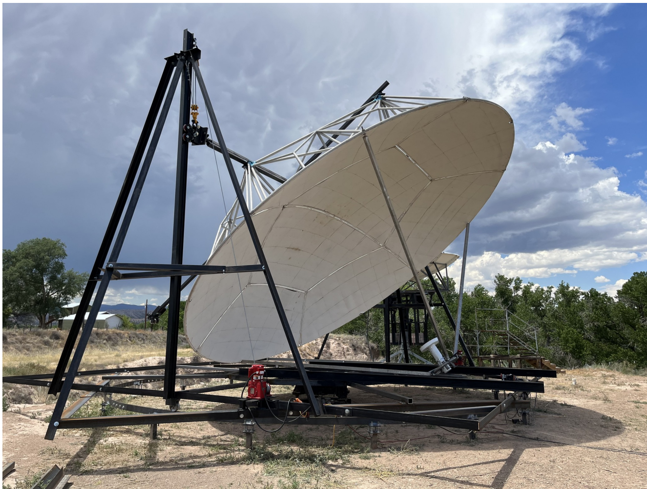
Figure 19. The dish has been tilted so that the feed horn may be straightforwardly installed from ground level (28JUL2023).
