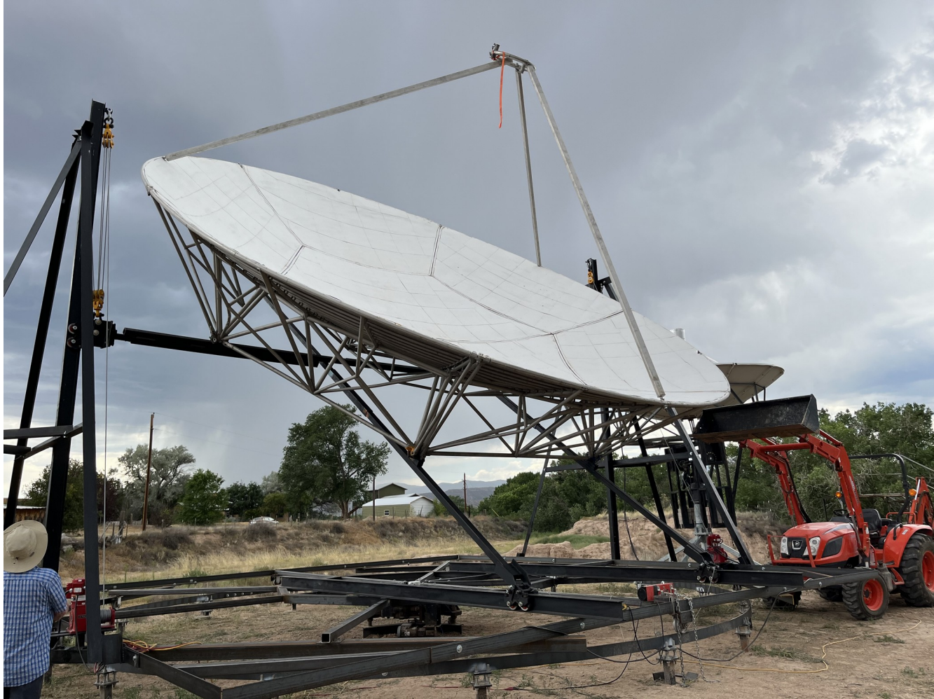
Figure 14. Dish being lowered into bird bath position with the broken-end support temporarily strapped to the mounting ring (27JUL2023).
