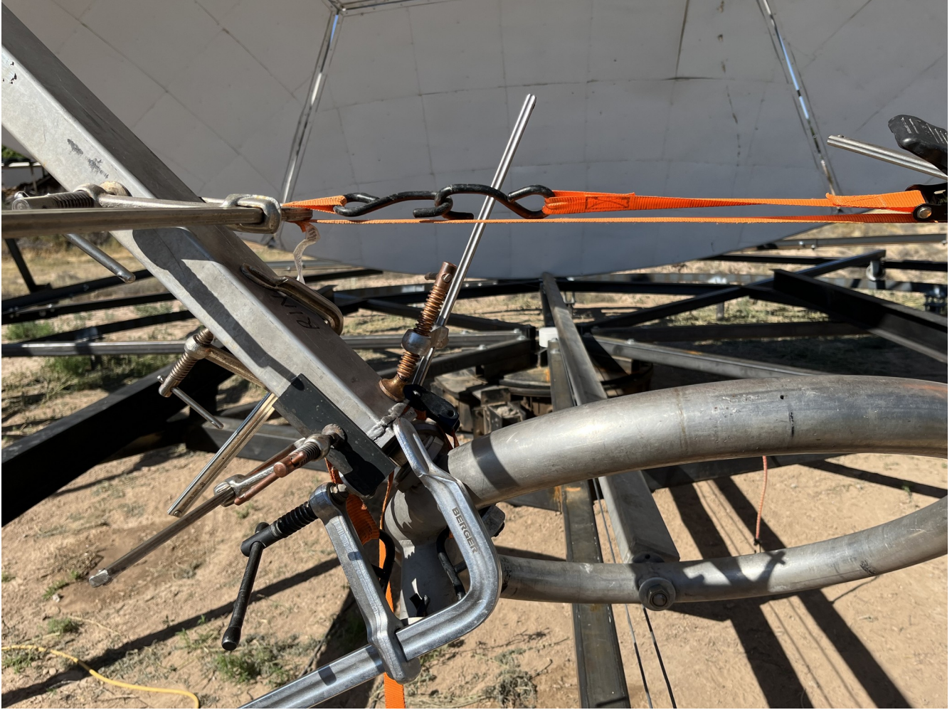
Figure 16. Multiple clamps and straps were used to hold the broken beam end onto the mating piece for welding (28JUL2023).
