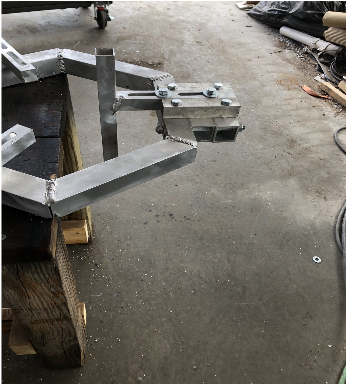
Figure IV-28. One side of an adjustable hexagon feed horn support assembly is now completed and installed, including welding an off-center cross member to the slotted support.
