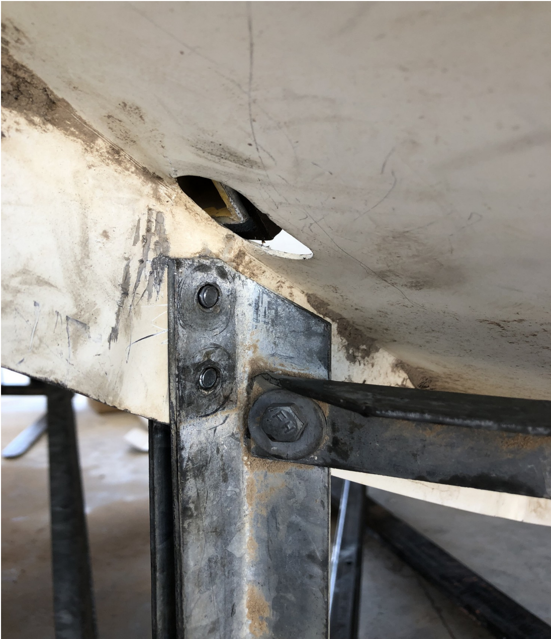
Figure IV-40. Under side connection point of the dish back structure to which the feed support arm bracket must attach.
