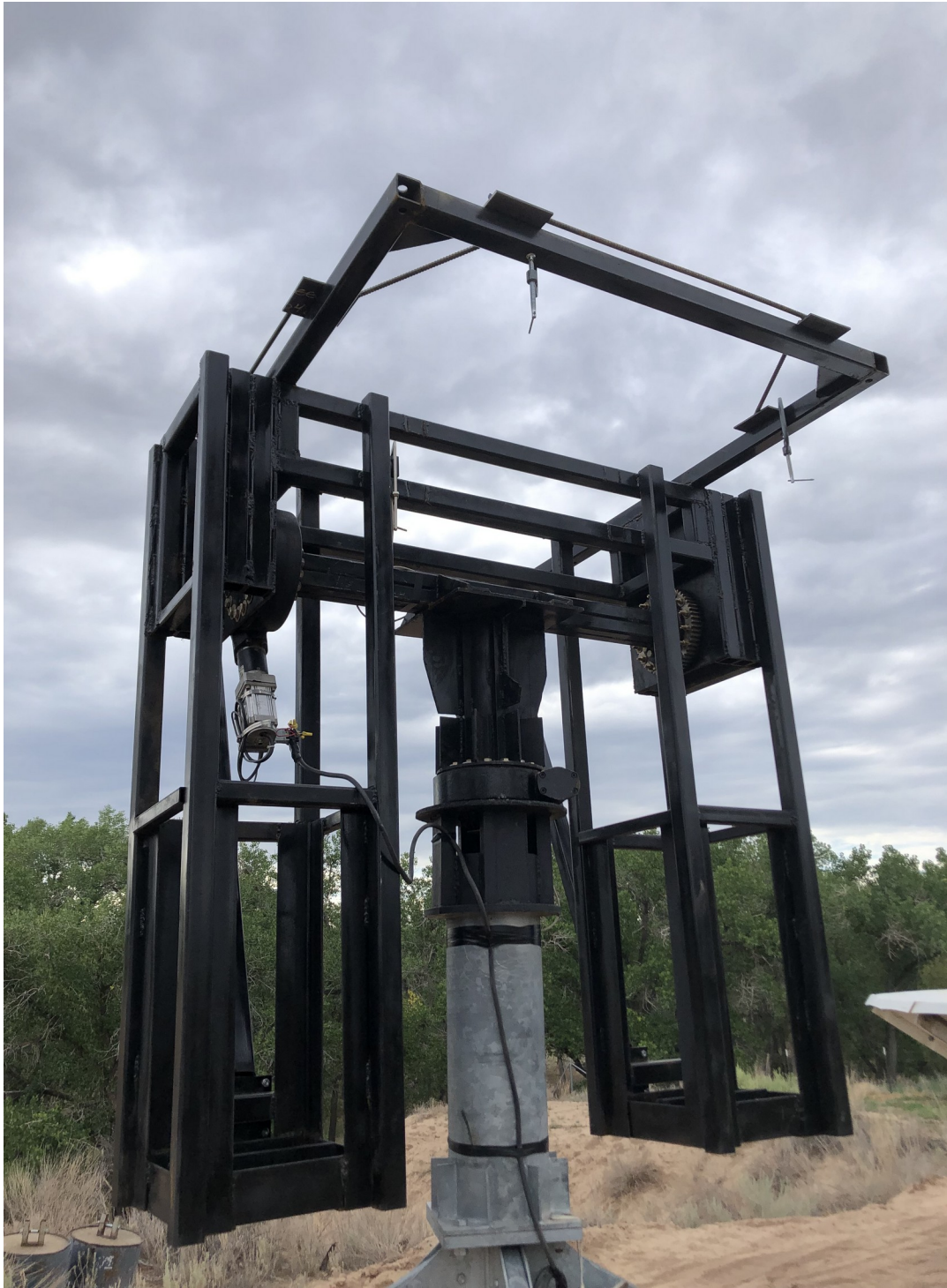
Figure IV-55. Rigid template completed and clamped onto the top member of the AZ/EL mount in preparation for hole marking and drilling.
