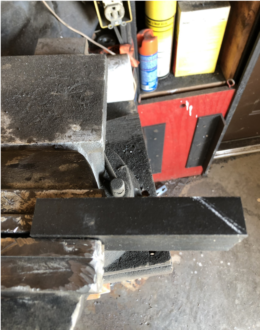
Figure IV-31. One of three bracket pieces marked for cutting of the required angle to be welded.
