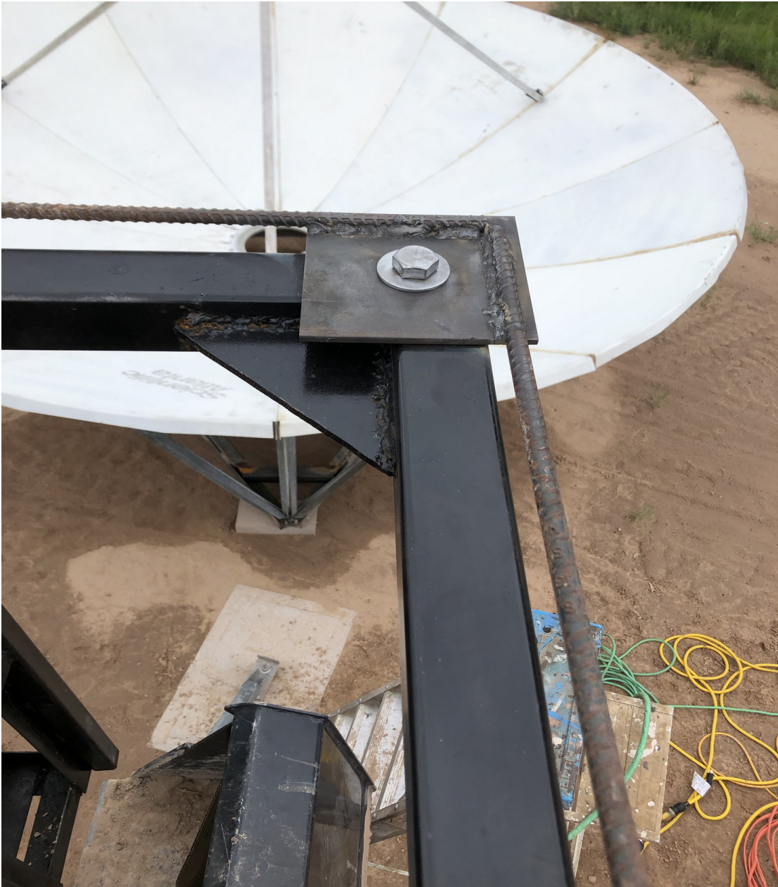
Figure IV-53. A corner of the rigid template after welding of two rebar connections.
