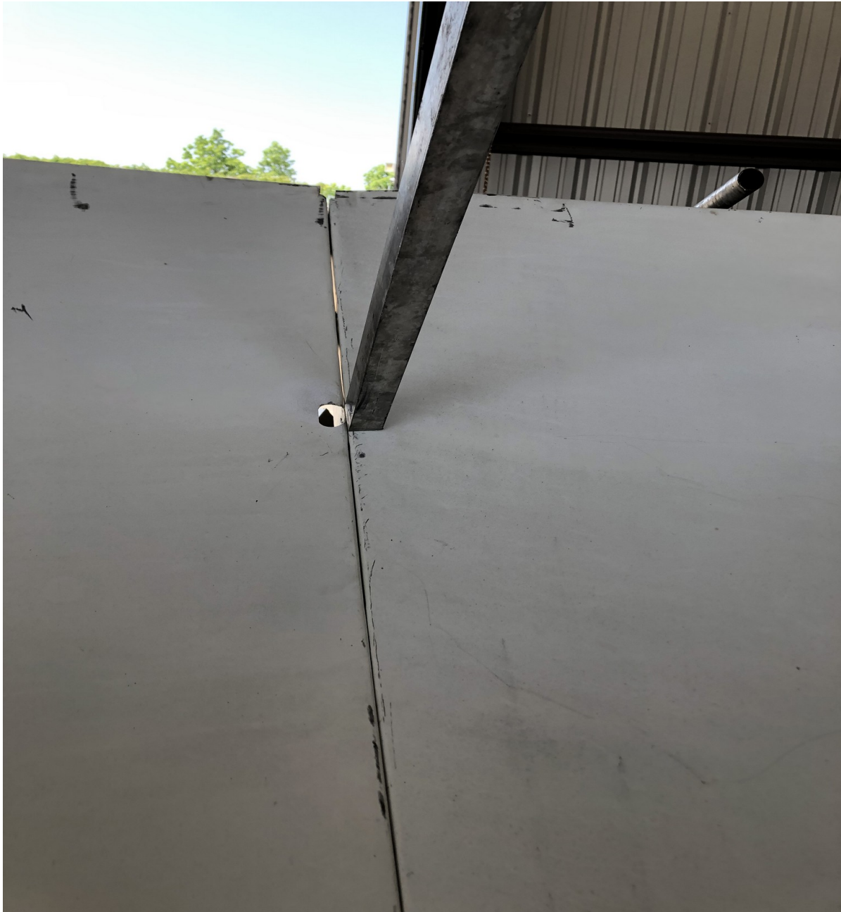
Figure IV-40. Lower end support arm positioning detail for fabricating and fitting of a lower end steel mounting bracket.
