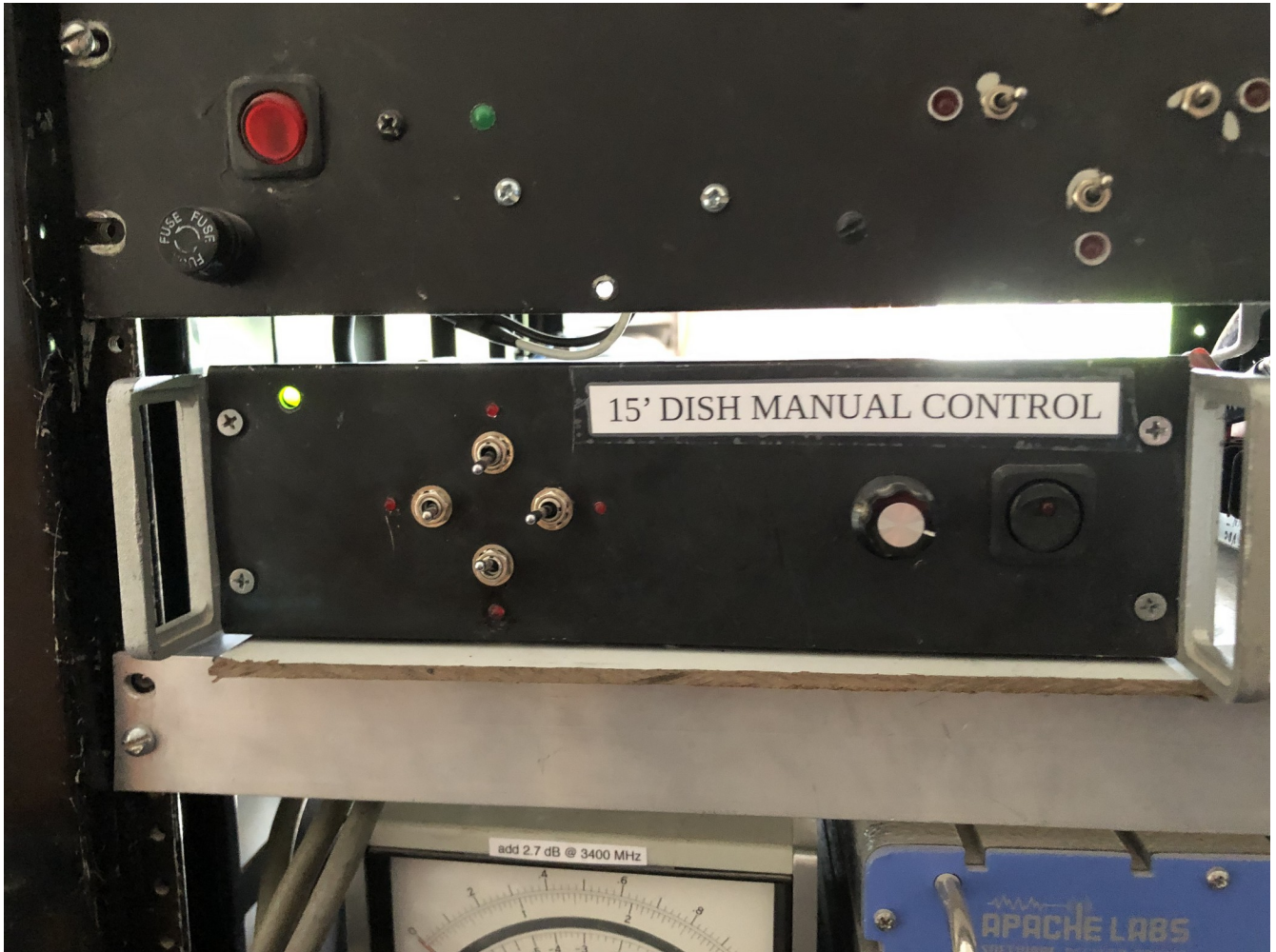
Figure IV-13. Front view of the dish motion control panel. The panel controls include manual motion control switches, an AZ motion speed control, LEDs that indicate when motion is in progress, and a panel power switch.
