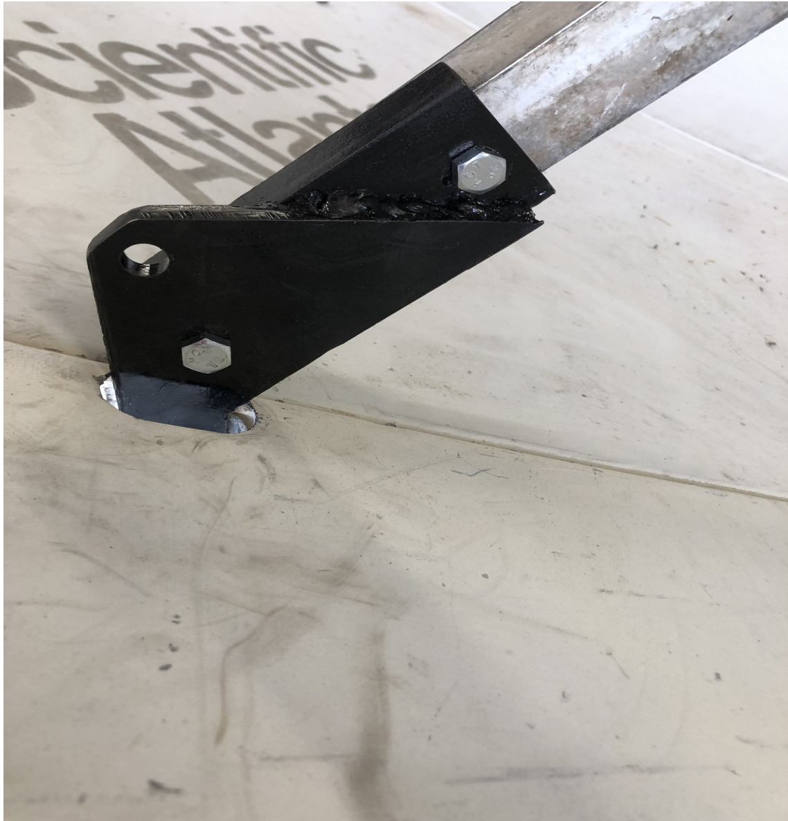
Figure IV-43. A completed lower end feed support arm bracket. Note the top hole that will be used to attach a clevis for assistance in lifting the dish later.
