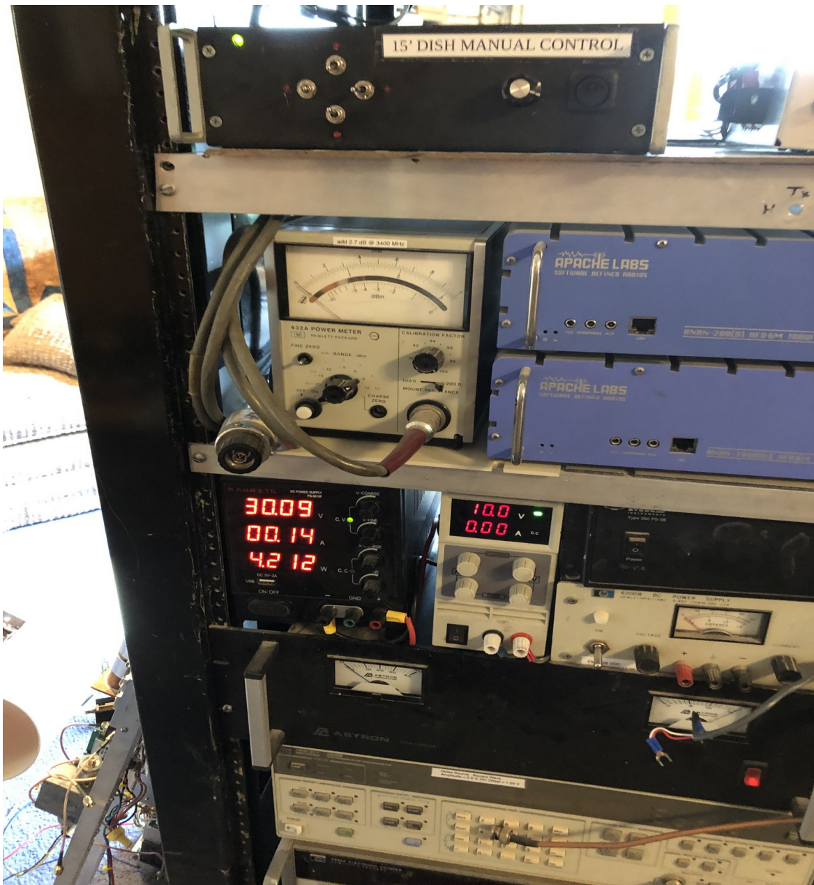
Figure IV-17. View showing the two external power supplies that supply operating voltages to the servo-motor driver modules of the AZ/EL mount.
