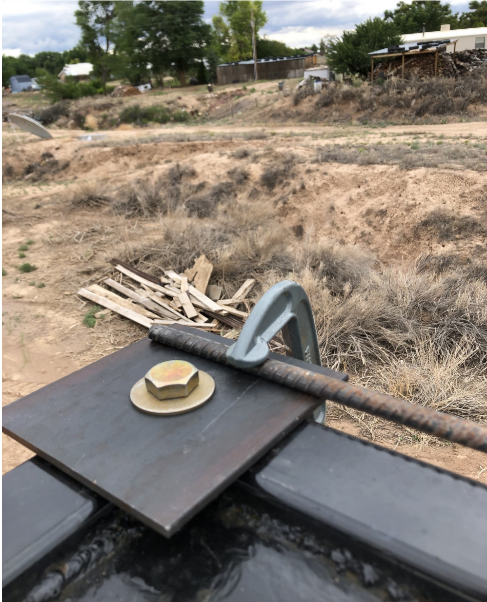
Figure IV-51. Rebar clamped onto a plate of the rigid template being fabricated prior to welding.
