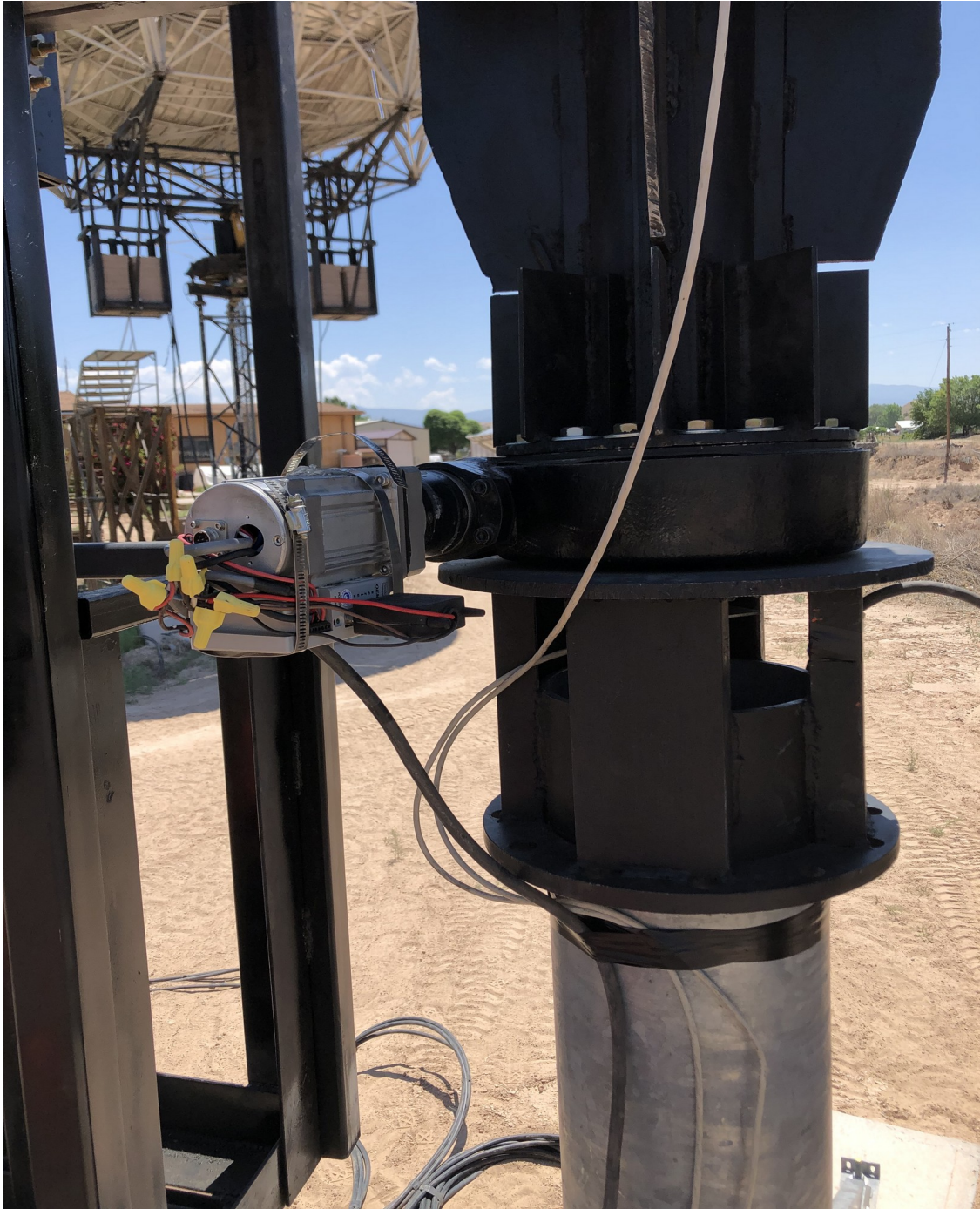
Figure IV-11. The AZ servo-motor driver module is strapped onto the AZ servo motor and temporarily wired to the AZ control lines from the telescope control room for testing and initial operations.
