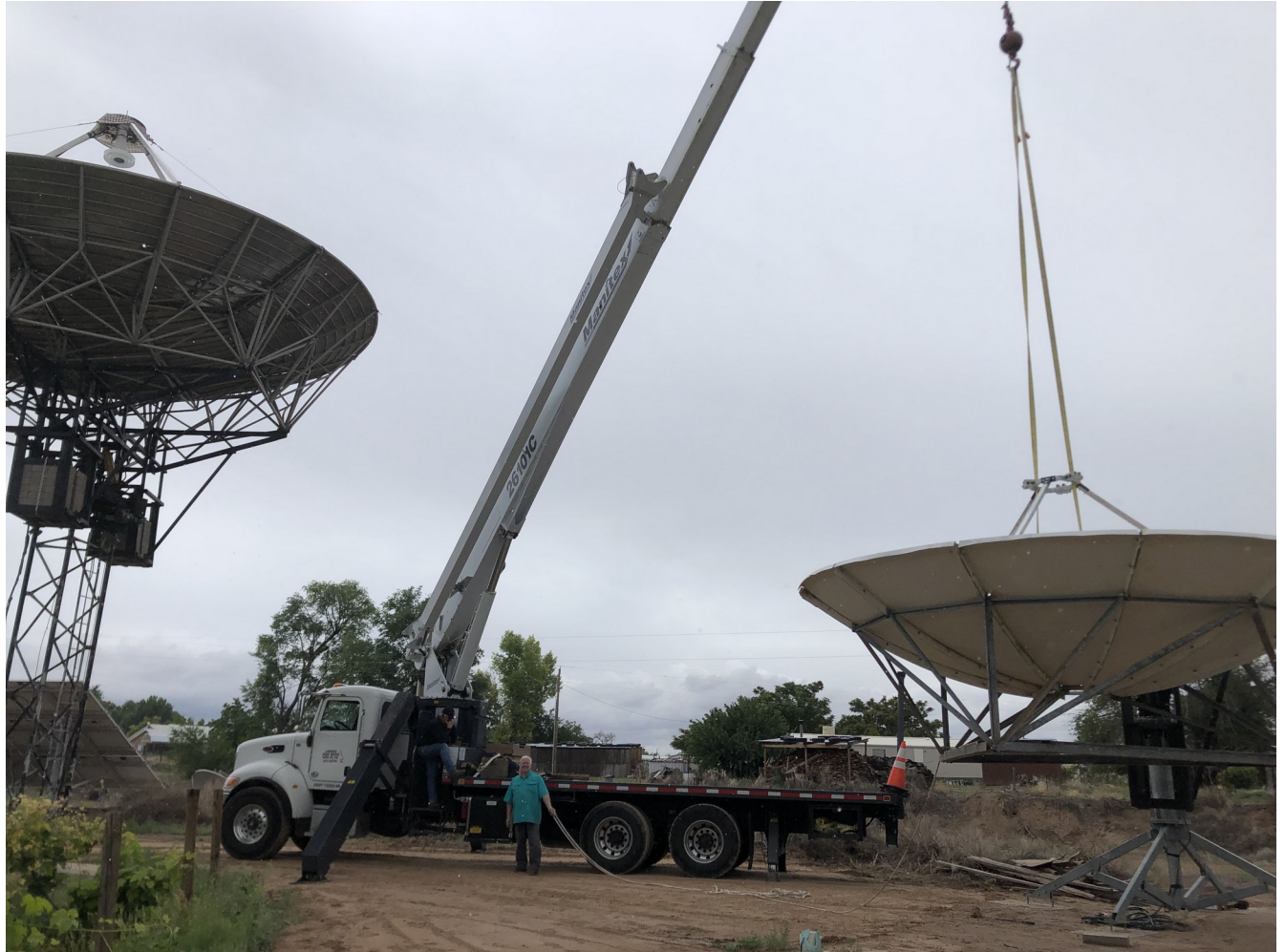
Figure IV-59. Test lift of the dish by the crane. Rigging and balance look good.
