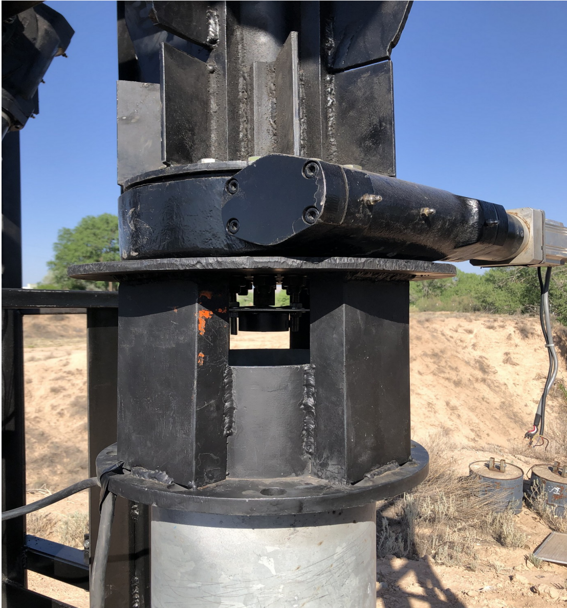
Figure IV-6. AZ encoder is installed.
