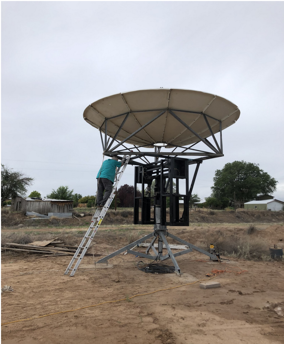
Figure IV-61. Bolt tightening after the dish was set onto the AZ/EL mount just as heavy rain began falling.
